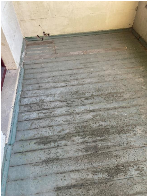
Figure 3 Original timber floorboards to the balcony of 99 Drummond Street Source: Stoll Architecture
