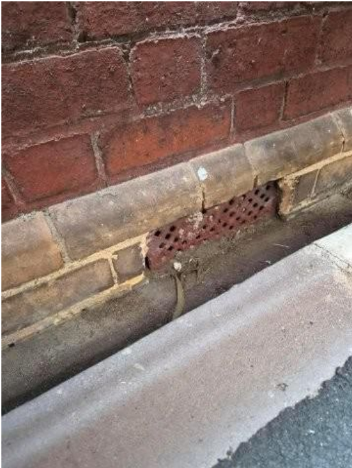
EXISTING VENT IN VENTILATION CHANNEL
