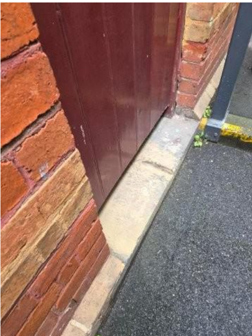
STONE SILL BENEATH STORE DOOR IN POOR CONDITION
