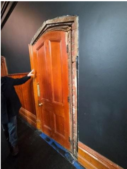
MISSING ARCHITRAVES AROUND STORE ROOM DOOR
