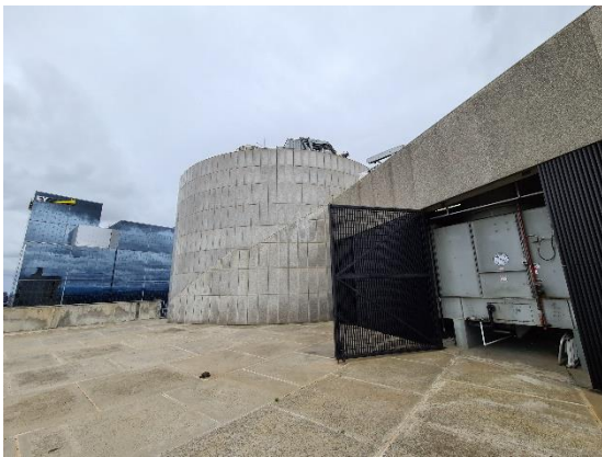
Figure 37 Plant enclosure at Level 29, and adjoining service core
