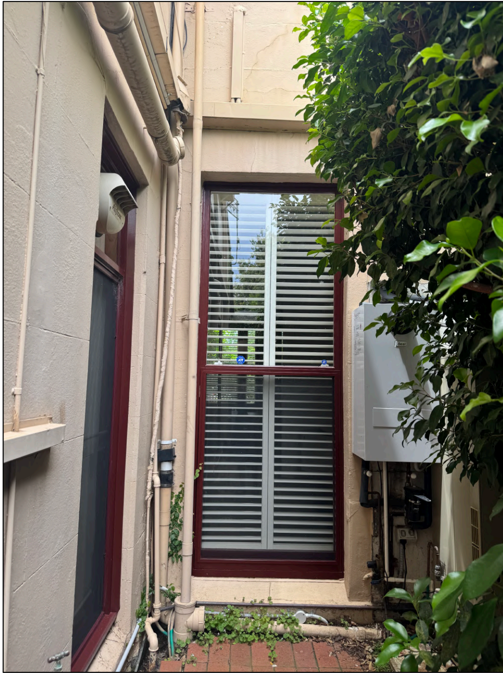
Figure 3 Altered window at ground level to the rear of the primary envelope. Modern connections (water, sewerage, electrical etc) are also evident attached to the rear wing.
