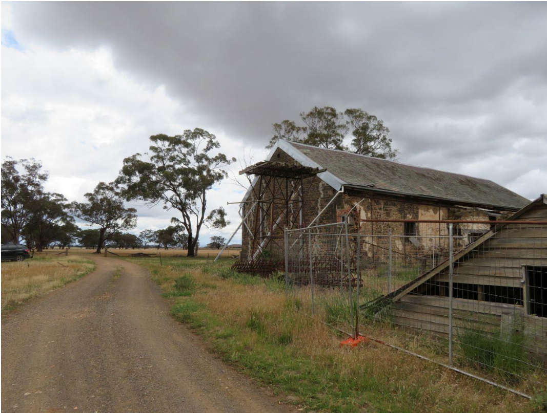
Figure 23 View to the underground tank (B11) (foreground) and south-east elevation of the barn/coach house (B10) (farm buildings precinct)
