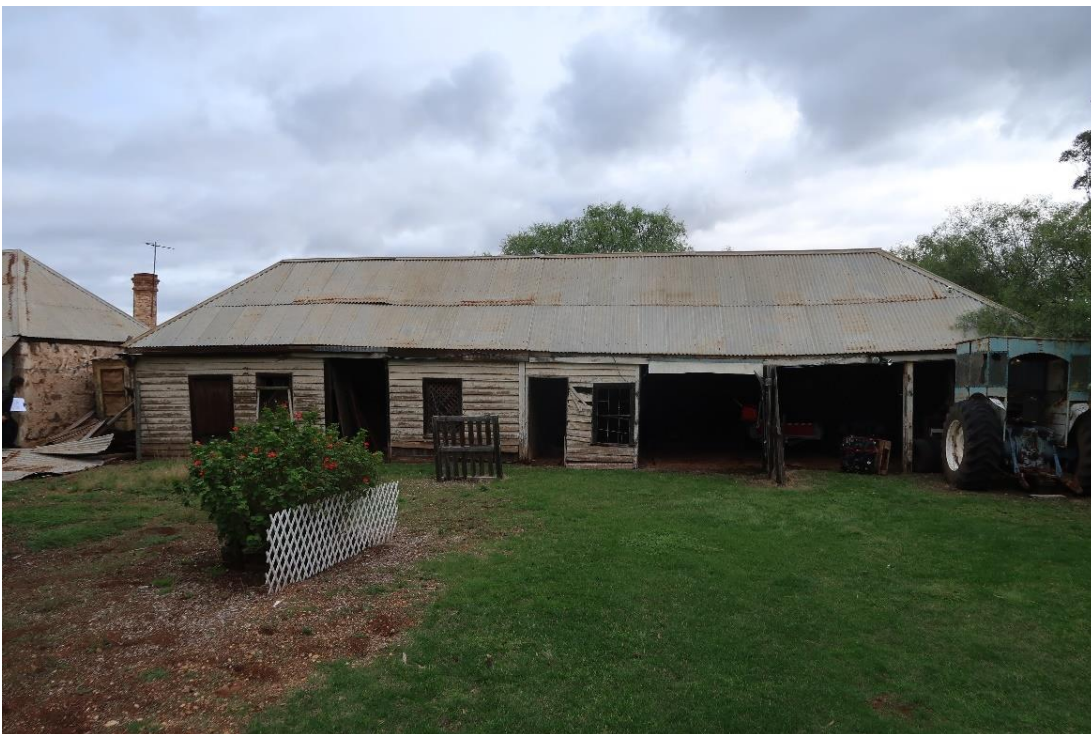
Figure 16 East elevation of the stable/garage (B4) north of the homestead (homestead precinct)
