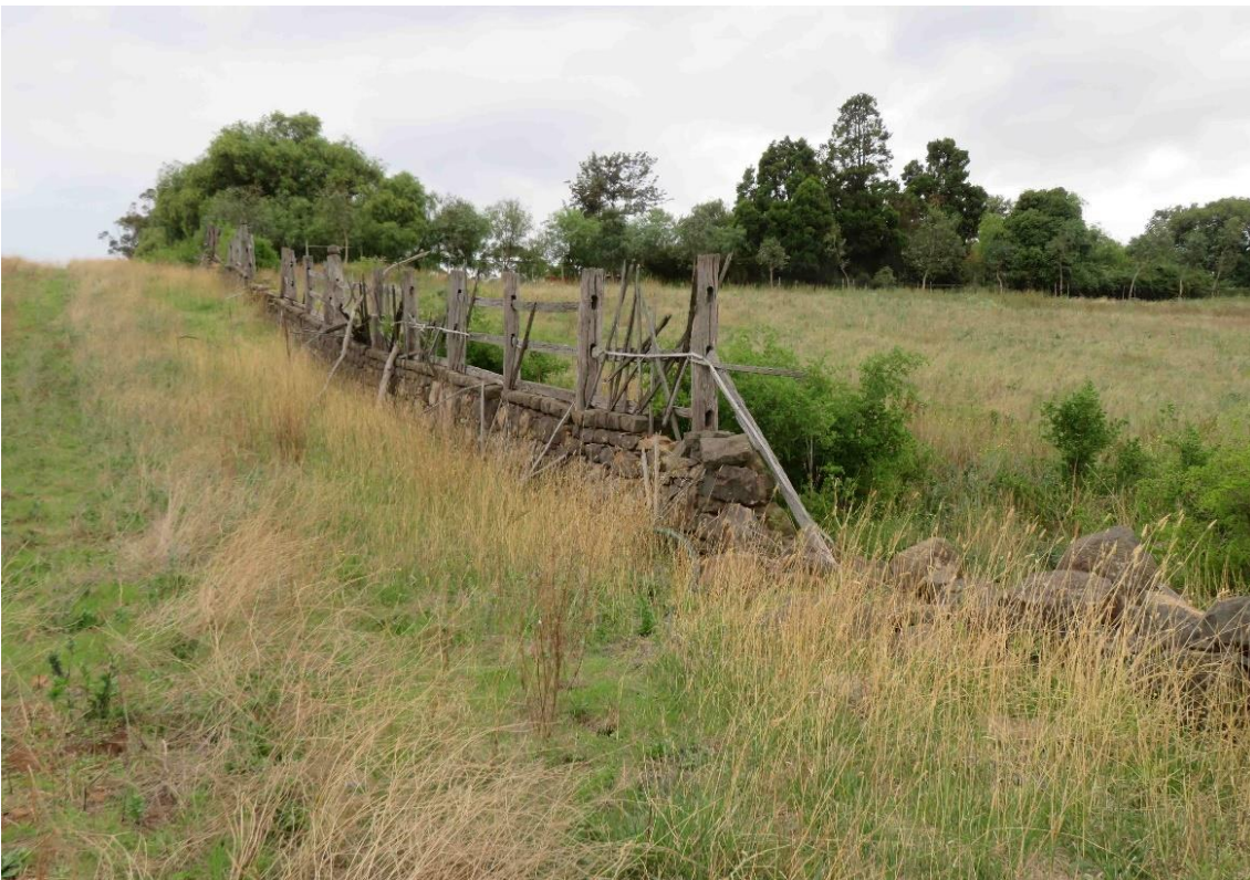
Figure 12 Southern extension of the bluestone wall with integrated timber post and rail fence (F3) (homestead precinct); some damage/loss of fabric is evident
