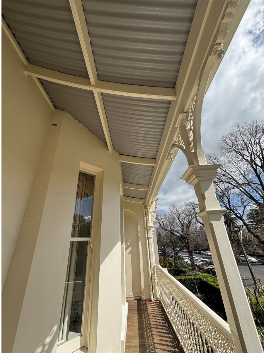
Figure 1 – The photo above shows overpainting of the original ashlar tooling. This is particularly evident on the left hand side of the first floor bedroom window.
