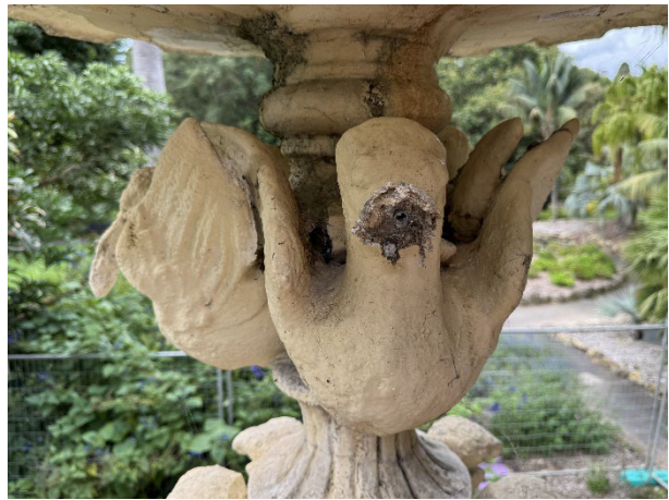
figure 10 – detail of one of the birds with the beak missing but the water pipe extant (2026)
