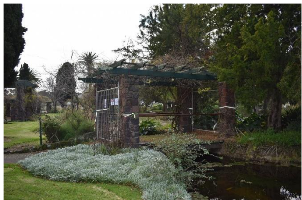
Figure 11. View of the timber arbor and bridge structure, currently under conservation works (source: Extent Heritage Pty Ltd, 2023).
