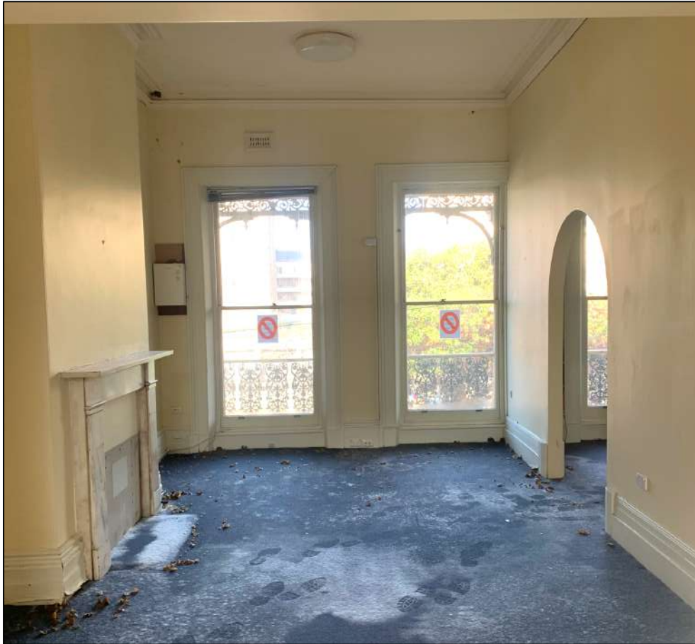
Figure 13 The original marble fireplace and significant recent mould growth present in the front room at level 1.
