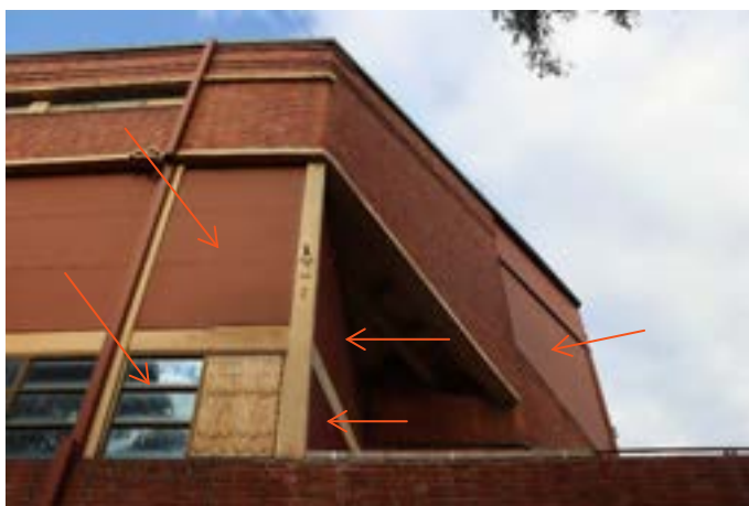
Figure 25: Detail lookup upwards at the southwestern corner showing infill (indicated by arrows), horizontal banding, non-original downpipe, concrete plats/soffit, and balustrade of walkway and stair emerging from promenade.
