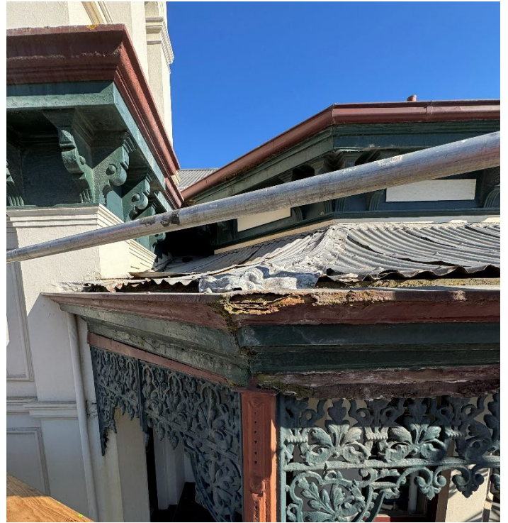
Figure 6 Rotten roof timbers and detached steel sheeting.
