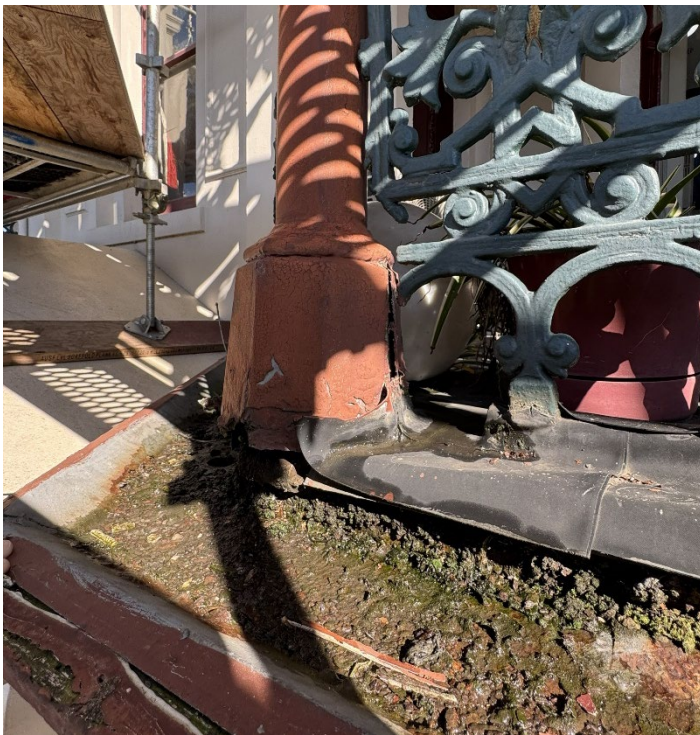
Figure 7 Split column base, rainwater system full of debris.
