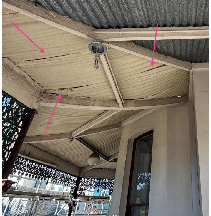
Figure 8 Splits in the first-floor soffit (indicated).
