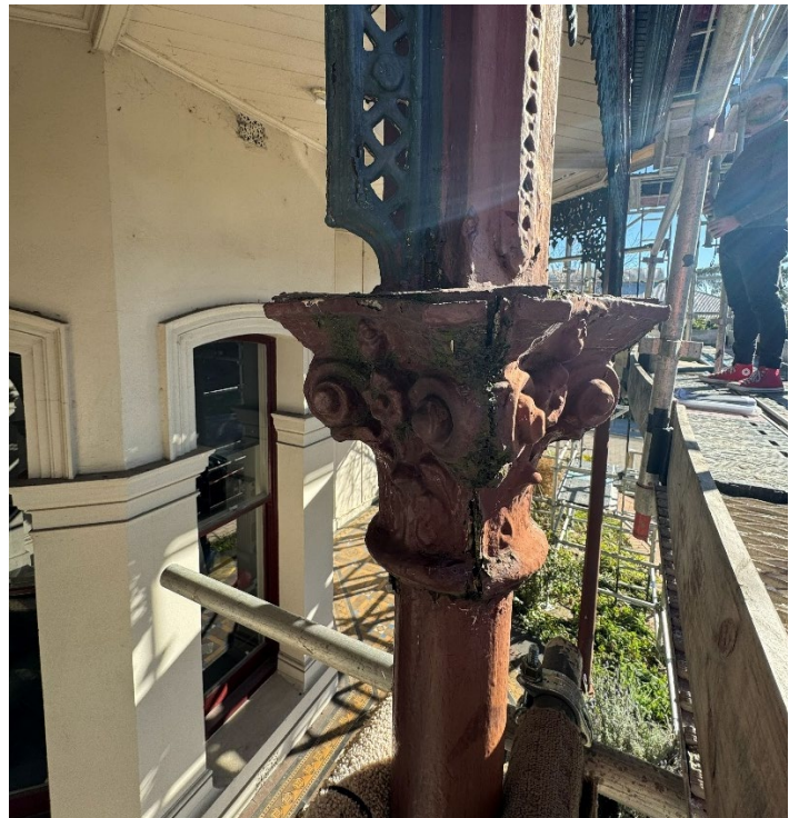
Figure 4 Damaged and degraded column post
