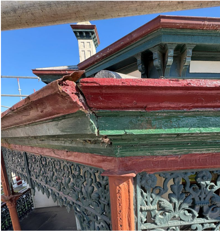
Figure 5 Misaligned roof timbers and detached capping
