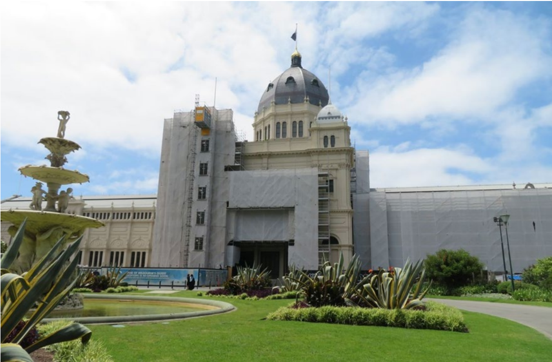
Figure 8 South façade of the REB c. 2019 during the 'Protection and Promotion' project
