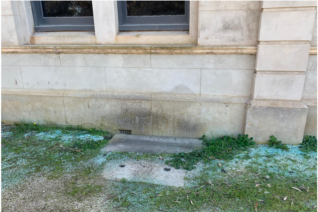
Figure 6 View of existing access to the sub-floor area of St Josephs Wing
