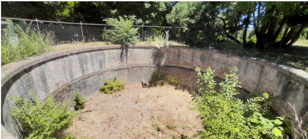
Figure 2.16 View of the Day Basin looking south, showing brick fabric, bluestone capping and a water pipe. (Source: GML 2022)
