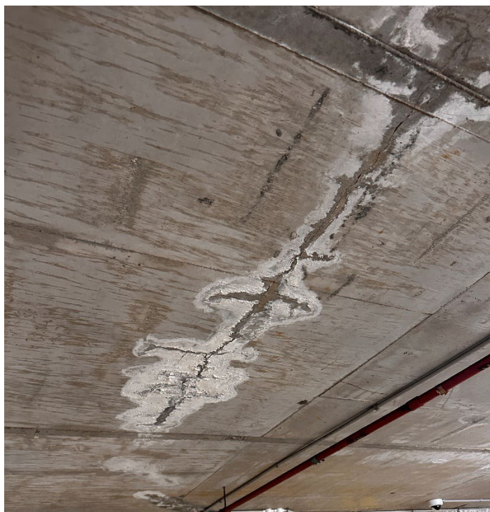
Figure 27 Leaking and efflorescence to carpark ceiling present in multiple areas, indicating continual presence of damp. These areas may be beneath garden beds.
