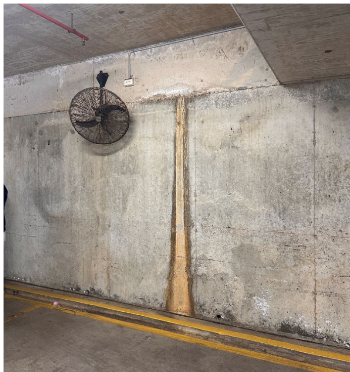
Figure 28 Concrete staining to carpark evinces water ingress through seams between concrete slabs.
