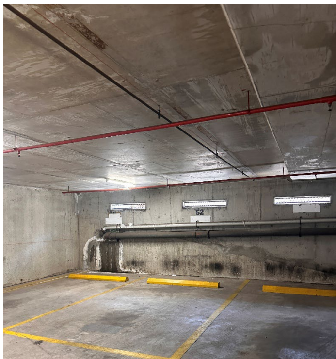
Figure 26 Efflorescence and staining to carpark walls may be attributed to presence of garden beds nearby and lack of waterproofing.
