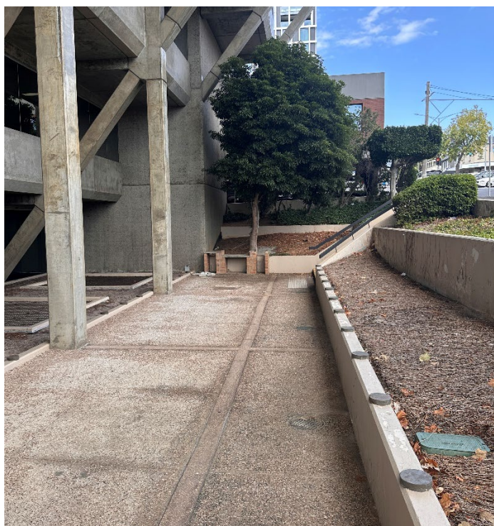
Figure 19 Fenwick Street lower plaza area. The pittosporum tree roots are damaging the planter walls and the barbecue is redundant.
