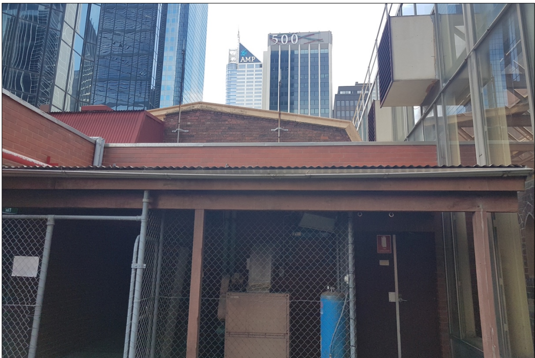
Figure 54 Current photograph showing modern roof top structure at the southern end of the Rialto Building.
