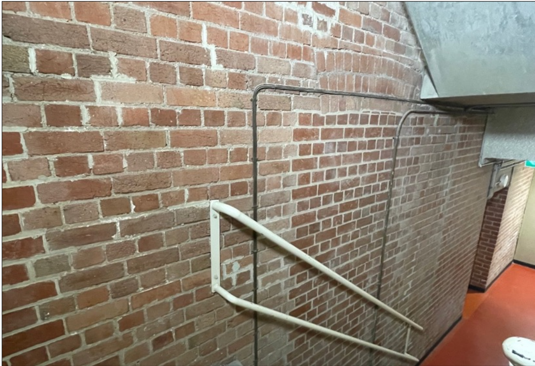
Figure 76 The south wall of the Winfield Building showing modern infill to original brickwork.
