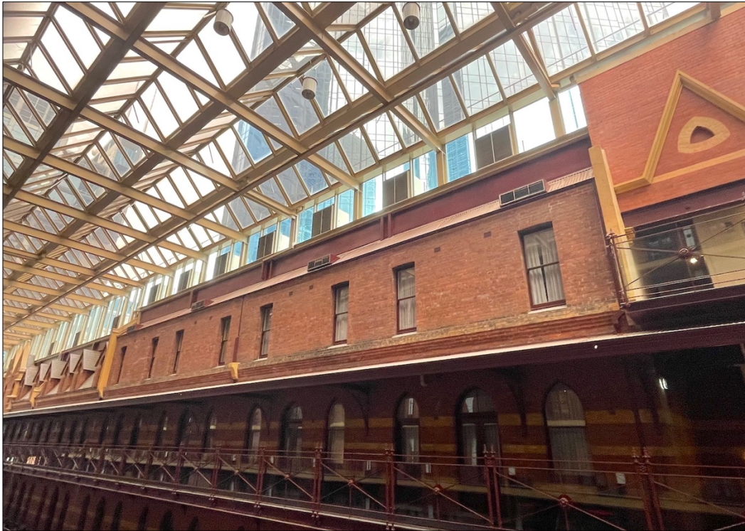
Figure 43 The northern end of the east elevation showing the 1904 wool exchange addition replacing the original slate roof with attic dormers.
