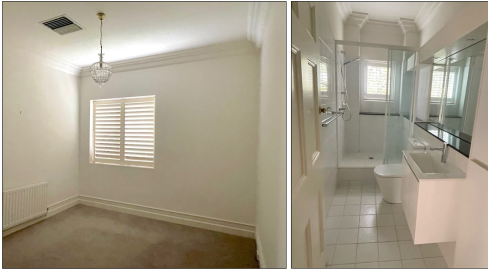
Figure 52 (left) First floor study, which was originally a bathroom. It has been stripped of all fittings fixtures and opened up to the east side by demolition of an internal wall.
