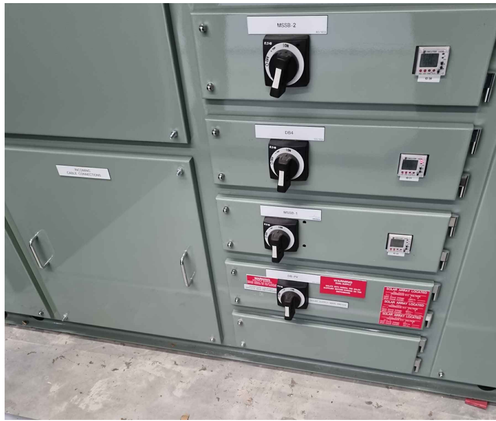
EXISTING MAIN SWITCHBOARD SPARE COMPARTMENT "EATON" BOARD
