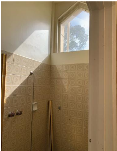
Figure 67 Current condition of G.112 and G.111
