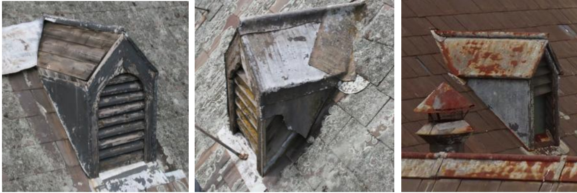
Figure 109 Various dormer vents showing failing lead cladding and rusting galvanised iron, ridge vent visible
