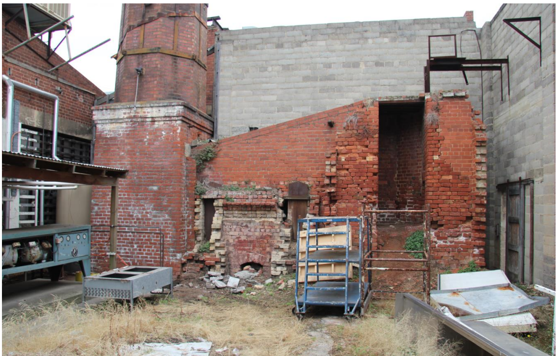
Figure 18 View of the fire tunnel remains and chimney prior to the demolition of the surrounding factory buildings Source: Lovell Chen archives, 2015
