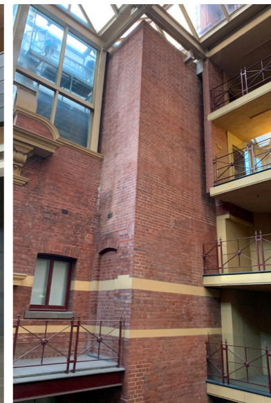
Southern wall of the Winfield. Upper portion of the wall added in the 1980's
