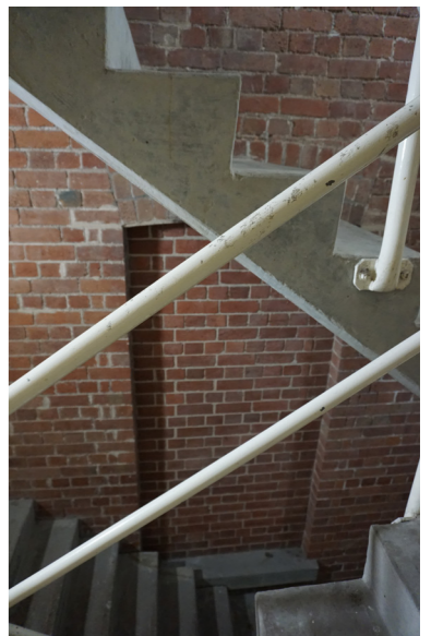
Photo of bricked up window on the Southern wall of the Winfield
