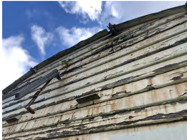
Figure 6: End elevations clad with splayed teardrop weatherboards. Boards typically in poor condition
