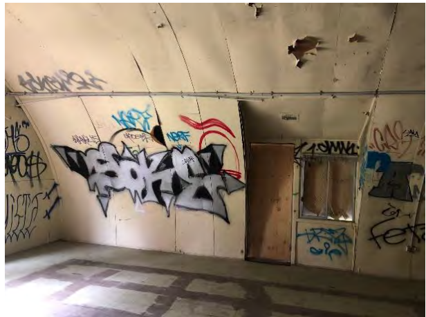
Figure 8: Internal Masonite lining in poor condition with extensive deformation and graffiti
