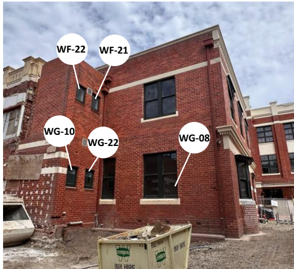
Figure 88: Subject site as seen from the northwest showing affected windows. Note that existing window between WG-22 and WG-08 has been approved under previous permit for conversion into door.
