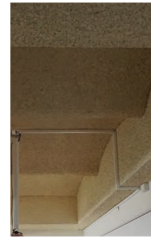
STATE OF ART FIRE PROTECTION
