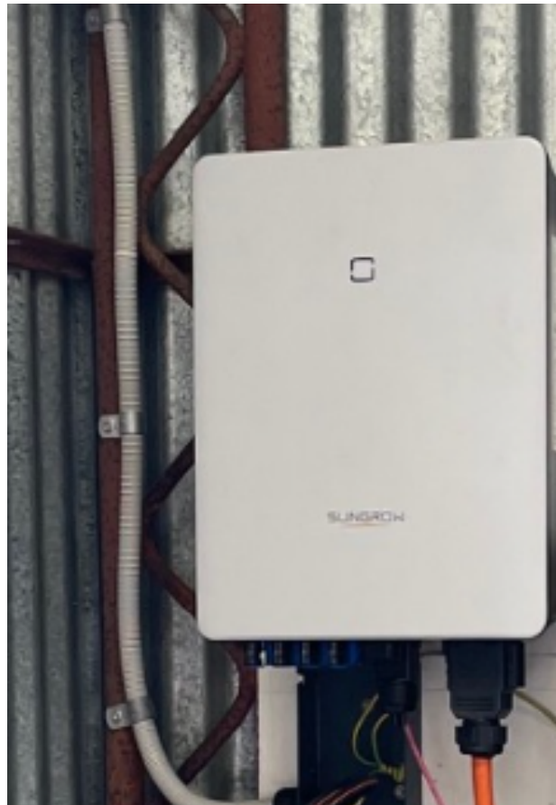
Photo 7. Photo of an identical inverter. This one is mounted on a wall of the Queenscliff Railway Workshops.
