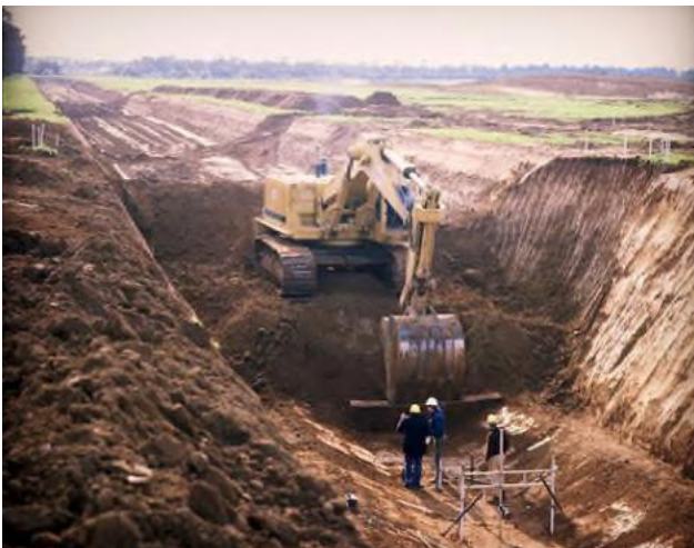
Figure 2-9: Construction of the WTS at Farm Road on 25 July 1983, facing east (Melbourne Water)
