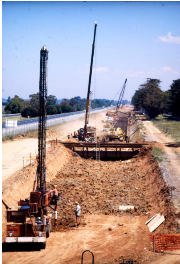
Figure 2-13: Construction of the WTS north of the Princes Highway (date unknown) (Melbourne Water)
