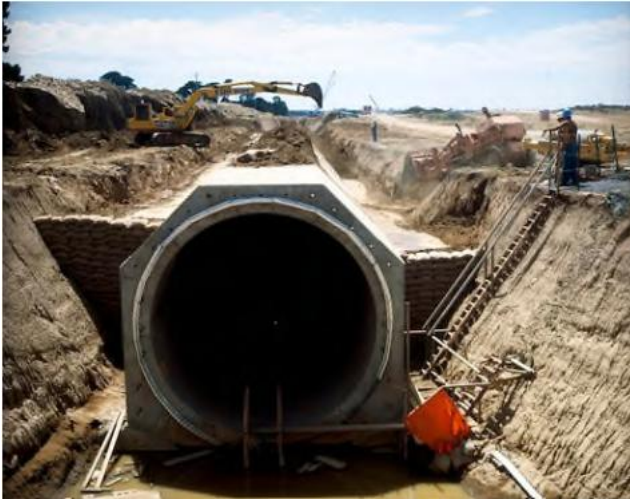
Figure 2-11: Back-end fill during construction of the WTS at Farm Road in February 1983 (Melbourne Water)
