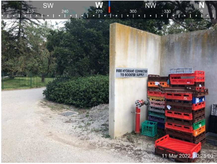
Figure 13: Location of new fire pump and water storage tanks, outlet adjacent to pool at north-western extent of Mansion grounds
