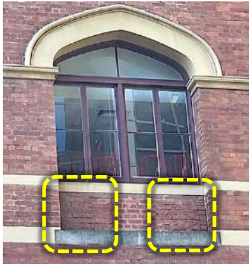
Indicative area where missing/degraded mortar is to be repointed
