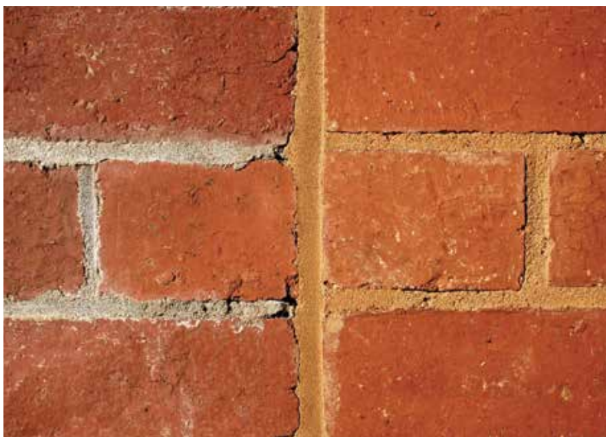
Figure 53: Nonmatching mortar. The new brickwork on the right uses a strong yellow sand, which does not match the original mortar on the left.
