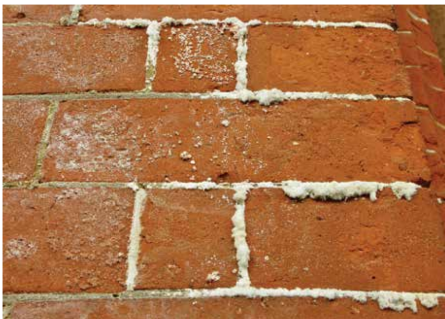
Figure 8: Permeable mortar. Salt crystals extruding from joints indicate that the lime mortar is more permeable than the bricks. By decaying in preference, and so protecting the bricks, the mortar is said to be sacrificial. Were the salt to be trapped in the less-permeable bricks, the damage to them would be very much greater than it is.
