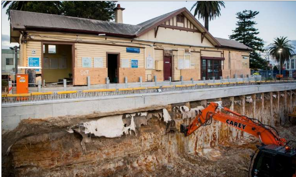
Figure 6 Excavation works for the level crossing removal occurring alongside the main station building, 2020.
