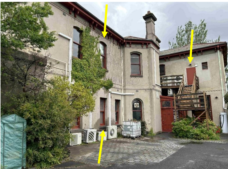
Figure 11 North elevation of Kwarau, showing the external fire stairs, timber airlock, pavers to be demolished; the services to be relocated as required; the windows and door proposed to be modified are indicated Source: Lovell Chen, 2025
