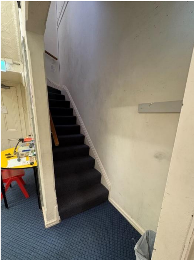
Figure 18 Existing non-compliant stair to be retained but made redundant and closed off Source: Bryant Alsop, 2026
