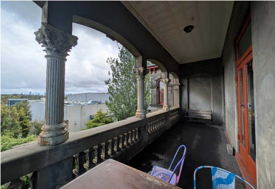
Figure 19 Existing original balustrades to the first-floor balcony; the glazed balustrade is proposed behind Source: Bryant Alsop, 2026
