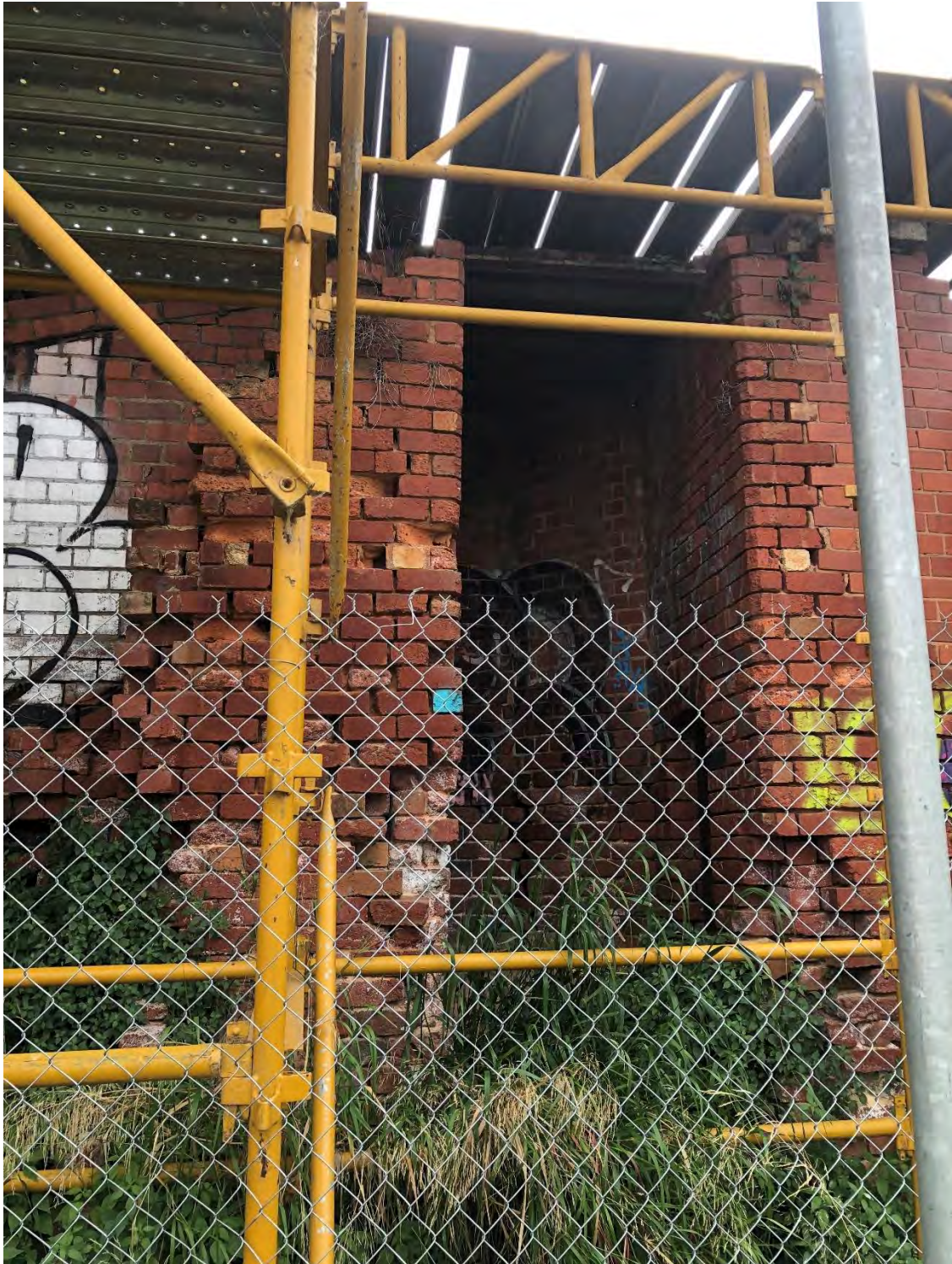
Image 2 – Existing Southern Walls showing previous alterations.
