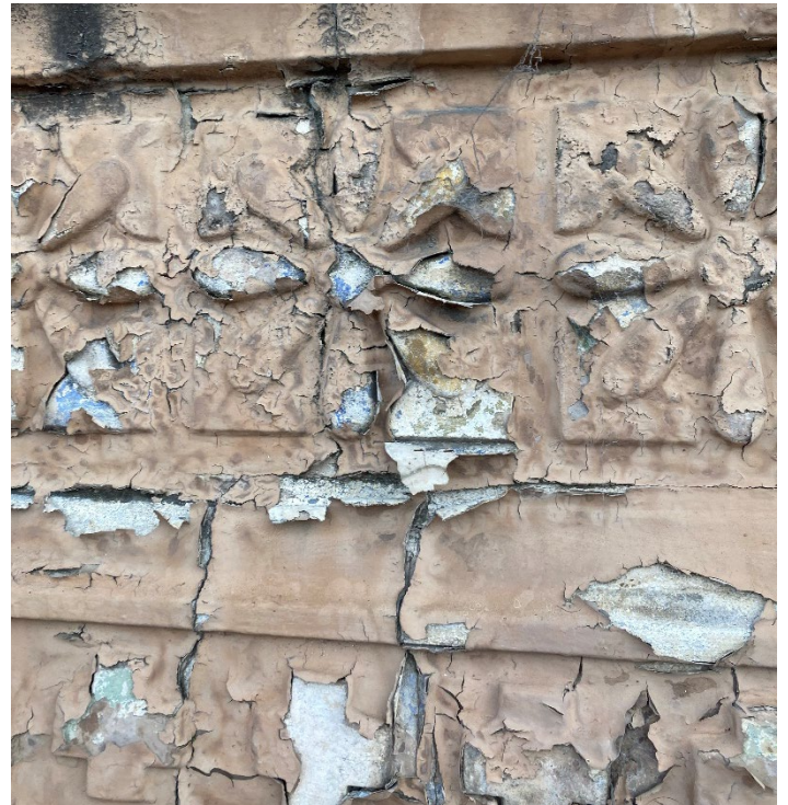
Figure 47 Typical flaking paint showing earlier colour schemes below the current paint system.
