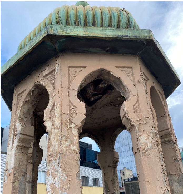
Figure 39 Corded and spalling ceiling to minaret on south elevations. Joints in concrete beginning to open.
