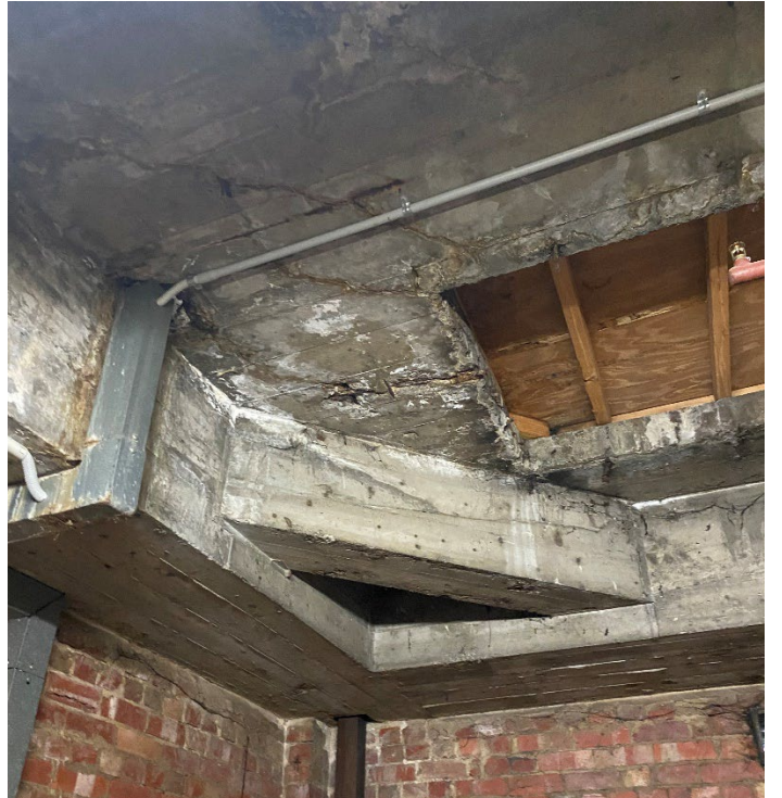
Figure 28 Salt affected concrete slab of the tower balcony
