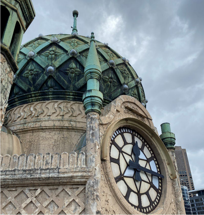
Figure 19 View of the clock tower. Note missing copper turret.
