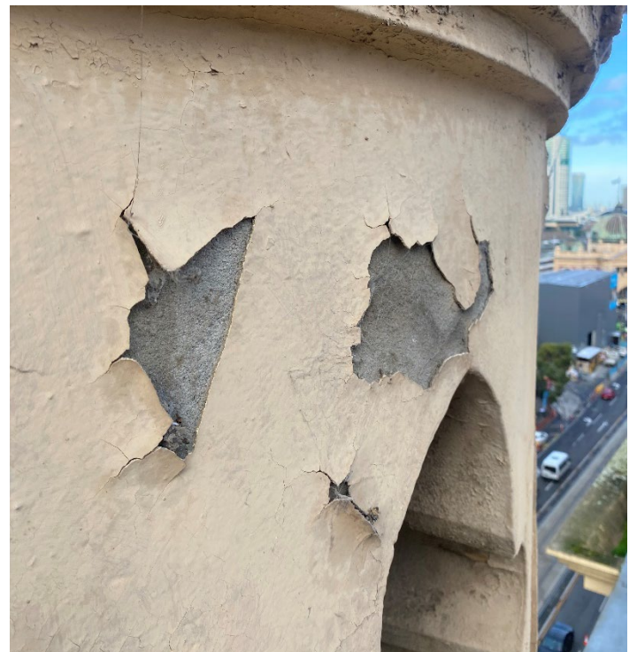
Figure 48 Peeling paint on the western minaret.
