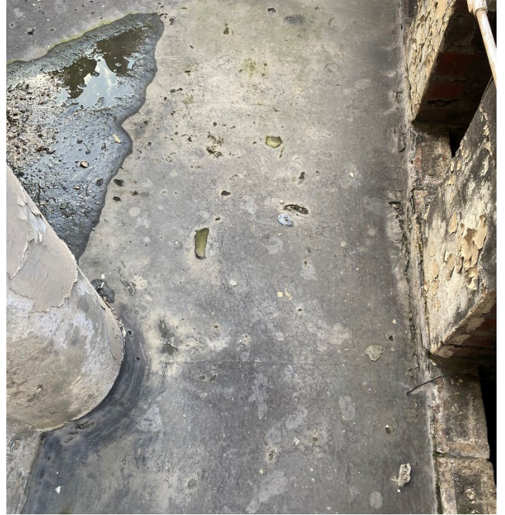
Figure 26 Defective membrane on tower balcony.
