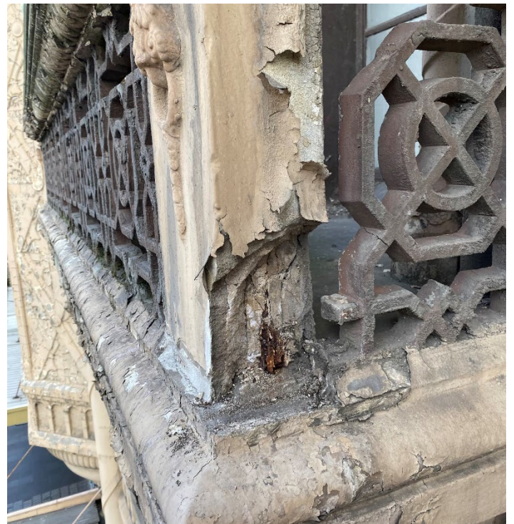
Figure 42 Spalling corner of the balcony balustrade piers.
