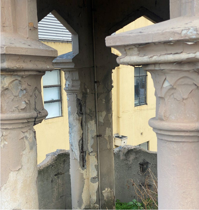
Figure 37 Spalling concrete post in minaret.
