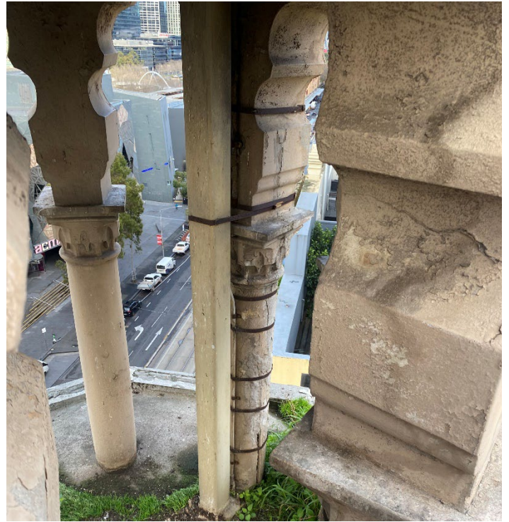
Figure 34 Typical 1980s repair of minaret columns with past and strapping.
