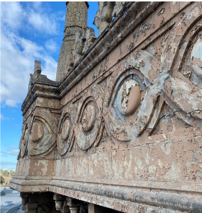
Figure 23 Cracking in the decorative reinforced concrete facing panels of the tower balcony.
