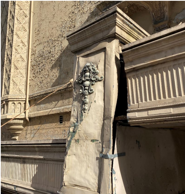
Figure 55 Impact damage to the canopy on Russell Street.
