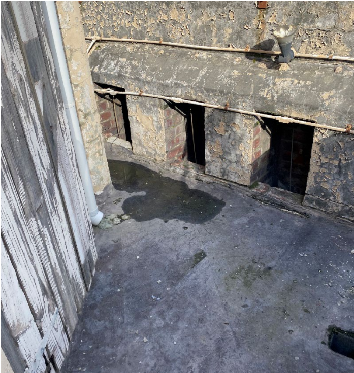
Figure 27 Defective membrane on tower balcony
