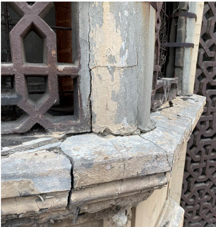
Figure 17 Spalling concrete structure on the canted by balcony.
