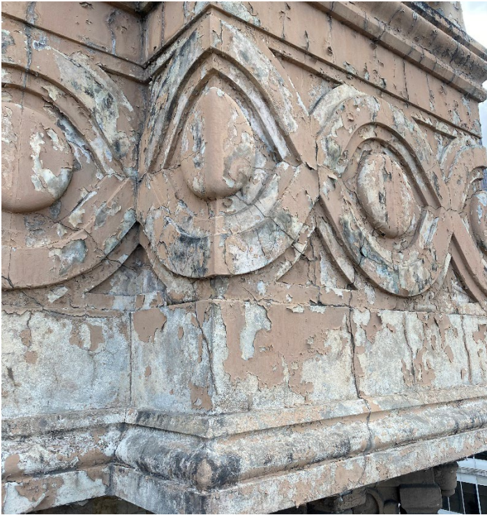
Figure 23 Cracking in the decorative reinforced concrete facing panels of the tower balcony.
