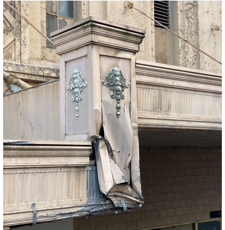
Figure 51 Impact damage to the canopy on Russell Street.
