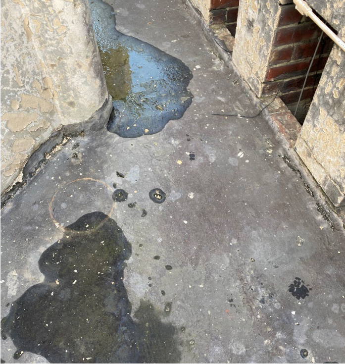
Figure 25 Defective membrane on tower balcony.
