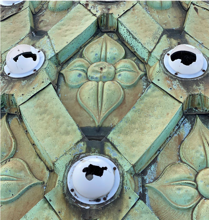
Figure 21 Detail of the onion dome showing broken light fitting covers.
