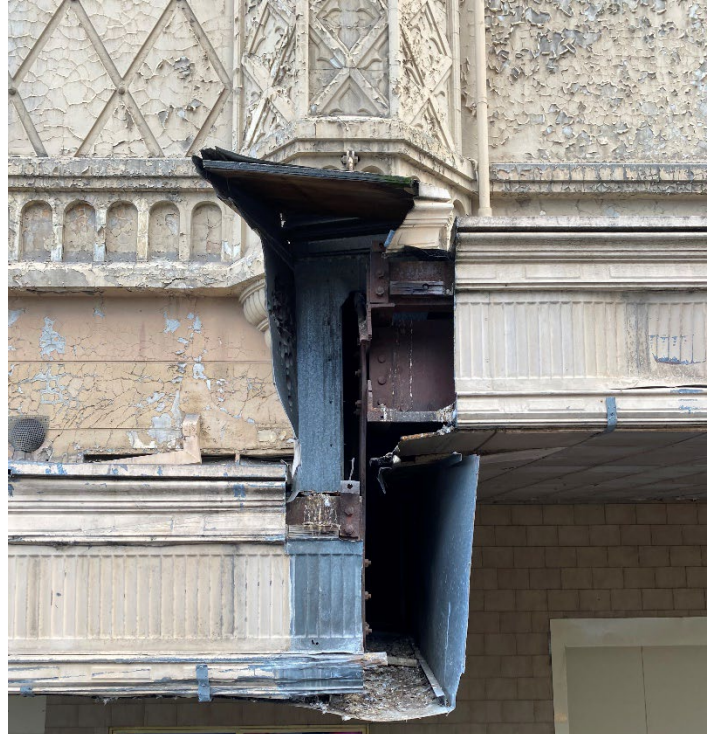
Figure 54 Section of missing and damaged canopy cladding showing the steel structure within.
