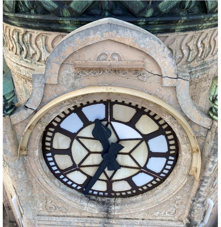
Figure 22 View of clock tower with crack through top of parapet.
