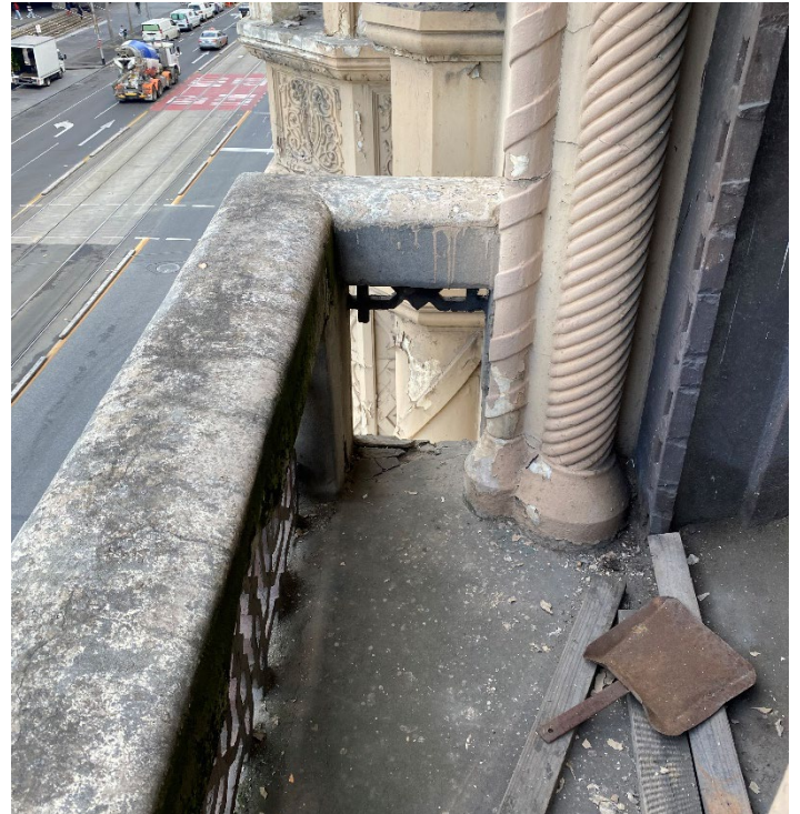
Figure 41 View of south elevation balcony with missing balustrade in end panel.
