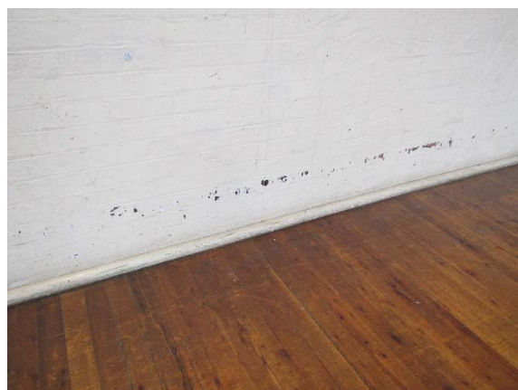
Figure 2.146 Damage to paint at skirting level.
