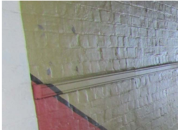
Figure 2.127 Detail of damaged paintwork in stairwell.
