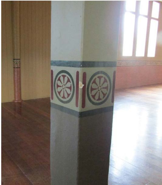
Figure 2.110 Chip to decorative scheme on column in southern nave.
