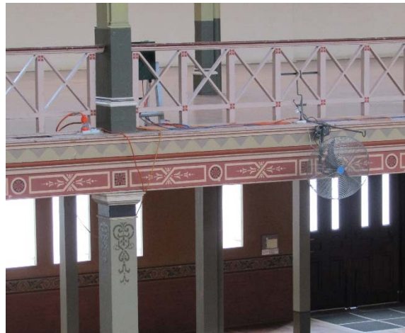
Figure 2.144 View of electrical fixtures and cabling.
