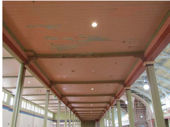
Figure 2.142 View of peeling paint in western gallery timber lined ceiling.
