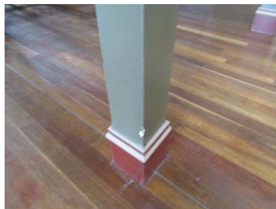
Figure 2.94 Example of damage at base of decorative post.
