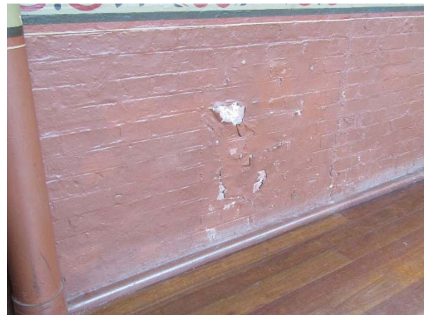
Figure 2.101 Detail of damaged paintwork.
