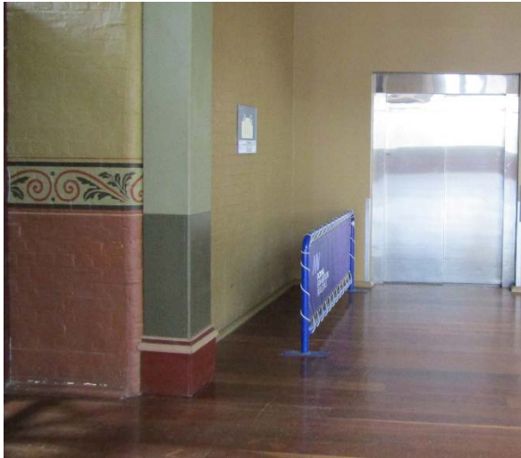
Figure 2.98 Paintwork adjacent to stair gates shows signs of abrasion at skirting level (lower left of image).
