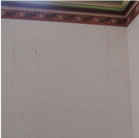
Figure 2.122 Penetrations and cracks evident in brickwork of north gallery wall.
