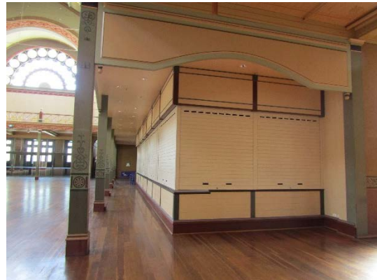
Figure 2.92 Kitchen/café area below northeast gallery. The decoratively painted posts are generally in good condition; however, there is evidence of both wear and tear and physical or other damage on some of the posts.
