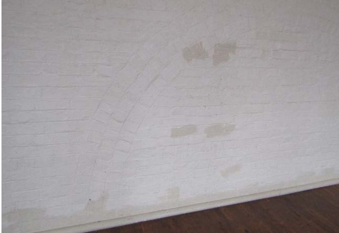
Figure 2.138 This lower section of wall has been repainted in several areas, suggesting physical or other damage to the paintwork. Other possible causes include water ingress and salt efflorescence (further investigation needed).
