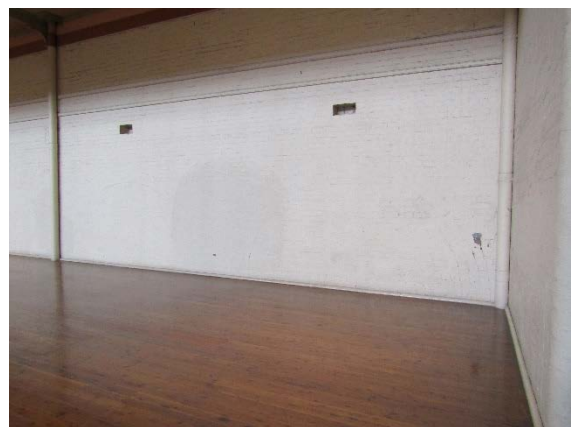
Figure 2.131 Mis-matched paint patching.
