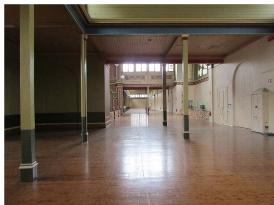
Figure 2.137 View along southern gallery. The replacement timber floor in this area is heavily marked.
