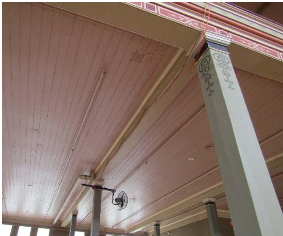
Figure 2.143 View of fixed hooks to underside of gallery to support electrical cables.
