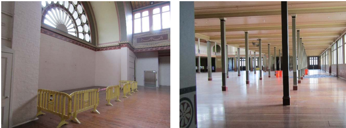
Figure 2.78 Remedial clean-up/maintenance due to water ingress.
