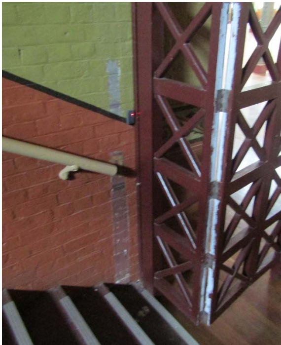
Figure 2.149 An earlier paint scheme (unprotected) is visible above the stair, adjacent to the gate, hinge is unpainted.
