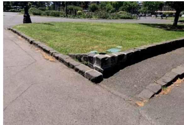
Figure 2.67 Eastern forecourt, proposed for VIP parking. Retaining walls are vulnerable to damage at ends and corners.
