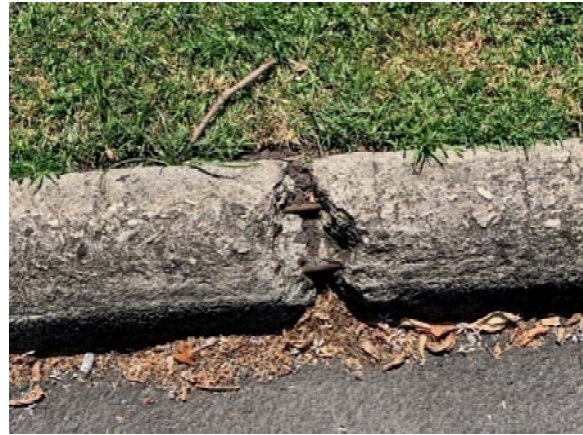
Figure 2.71 Concrete edging to carriage loop at east forecourt shows damage at joints, exposed reinforcing.
