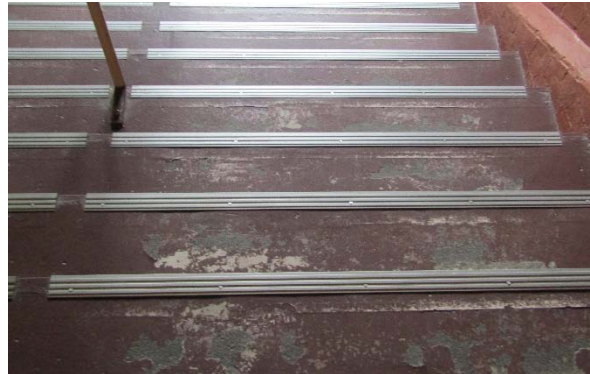
Figure 2.148 Worn paint surface to stairs leading to western gallery.
