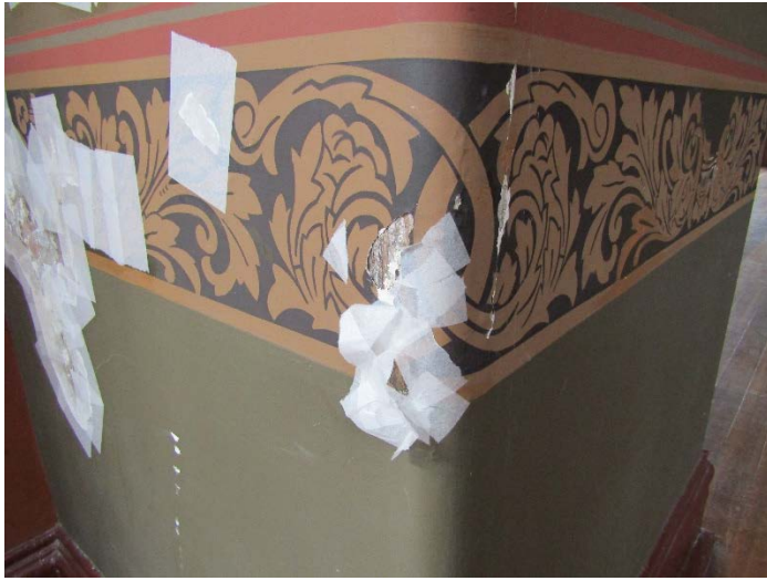
Figure 2.85 Detail of conservation works to damaged frieze, and damaged paint below.
