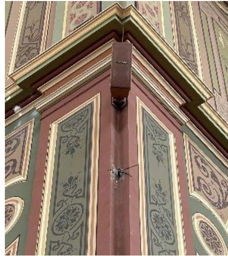
Figure 2.86 Exposed wiring visible on a central pier.
