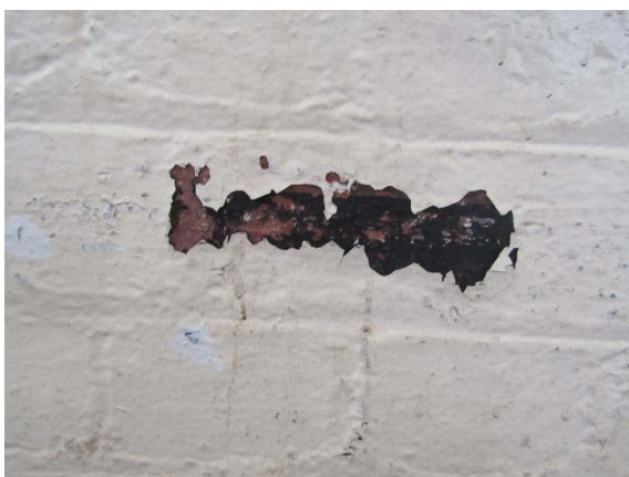
Figure 2.145 Example of paint delamination.
