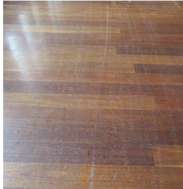
Figure 2.111 Evidence of linear scuffing and scratches to floor near southern nave.
