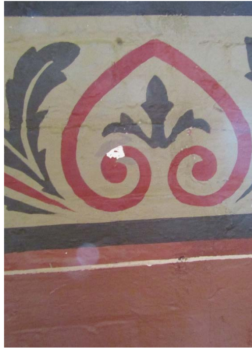
Figure 2.119 Chip and paint patch in decorative frieze.
