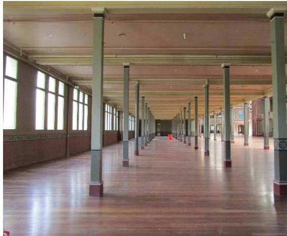
Figure 2.107 Flooring of side arcades is generally in good condition, some signs of scratches, scuffing and wear and tear.
