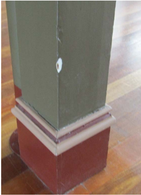
Figure 2.118 Chip to corner of lower section of painted decorative post.
