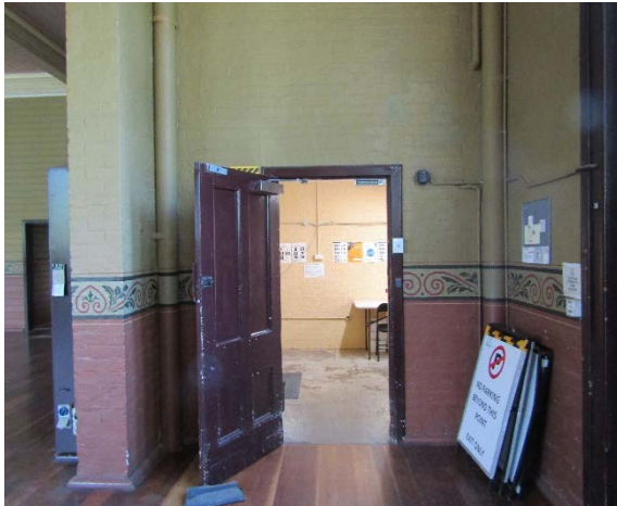
Figure 2.106 Evidence of vulnerability and paint damage around utility areas.
