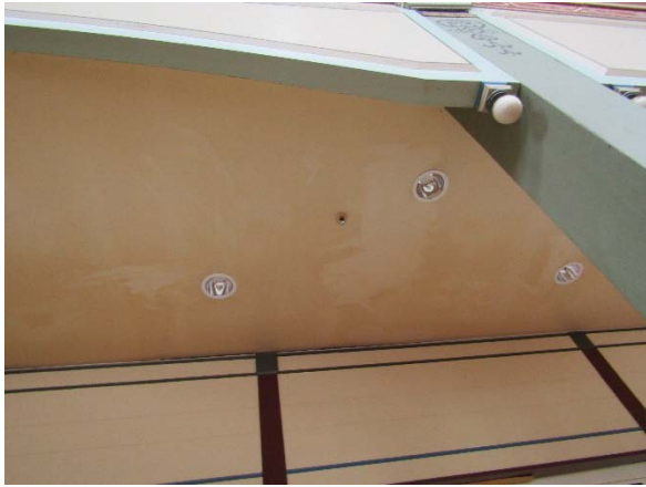
Figure 2.95 Discoloured paintwork visible on ceiling below northeast gallery.
