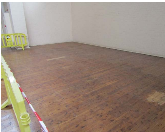
Figure 2.124 Evidence of patch repairs visible.
