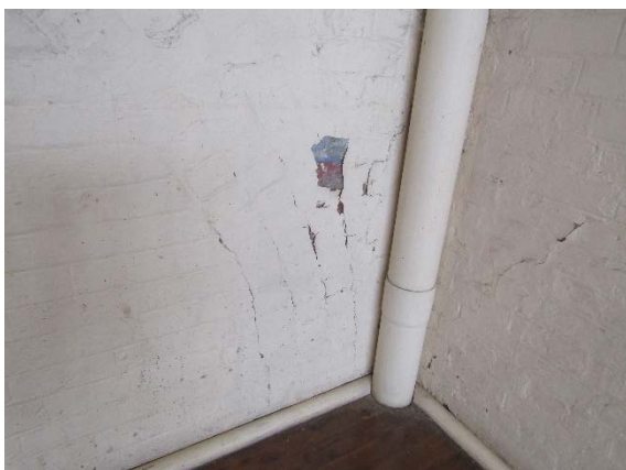
Figure 2.130 Detail of delaminating paint.
