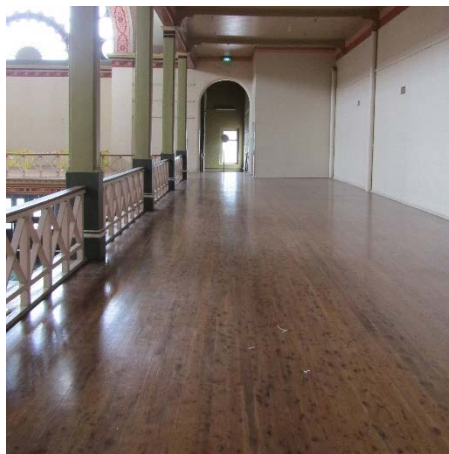
Figure 2.125 The timber floor is in generally sound condition; however, some areas of the gallery are quite worn with patch repairs visible.
