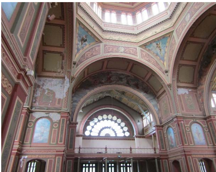
Figure 2.79 The decorative scheme is generally in good condition, with some conservation works still to be completed.
