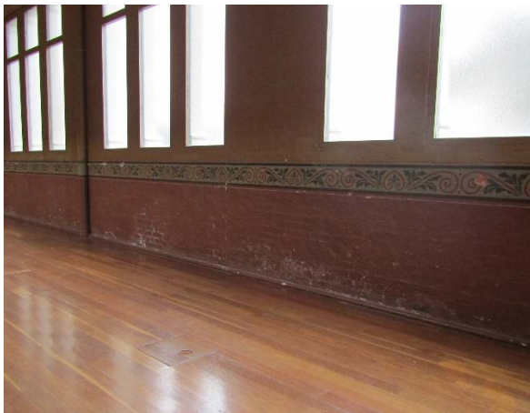
Figure 2.100 Walls are generally in good to fair condition, with some signs of wear and tear. The lower section of wall shows possible signs of water damage and salt efflorescence (further investigation needed).
