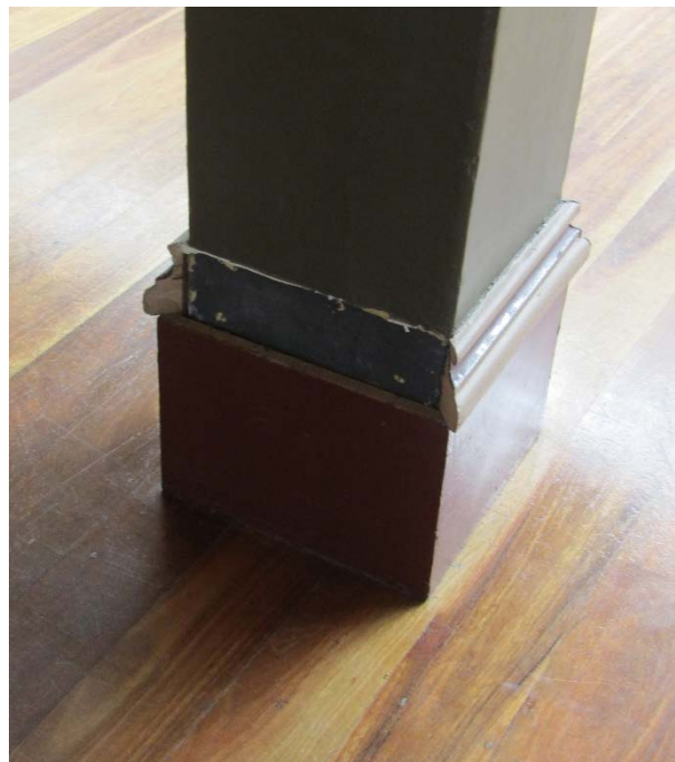
Figure 2.117 A section of skirting beading profile is missing from column base.
