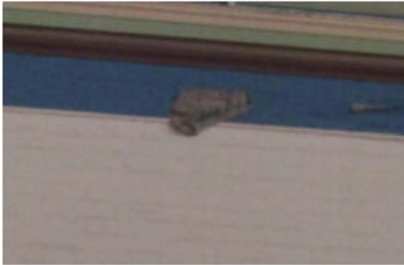
Figure 2.147 Detail of paint delamination on frieze band below clerestory window.
