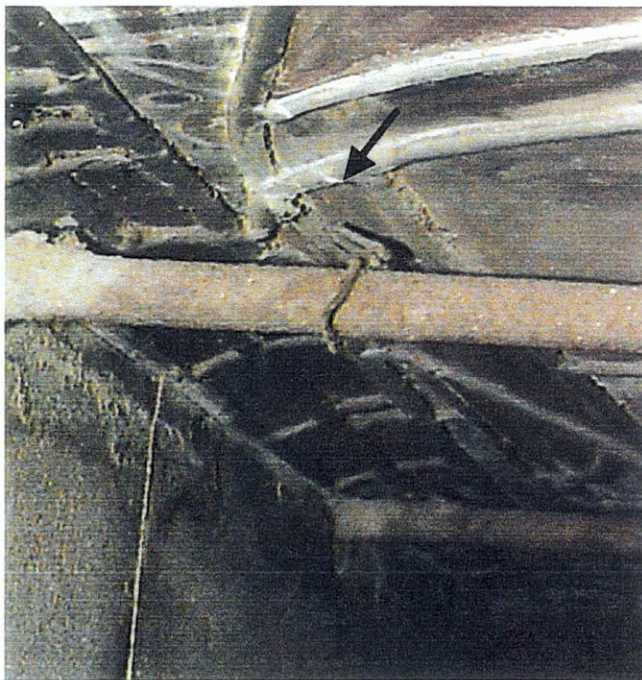
Vertical buckling and broken tie wire, St. John window
