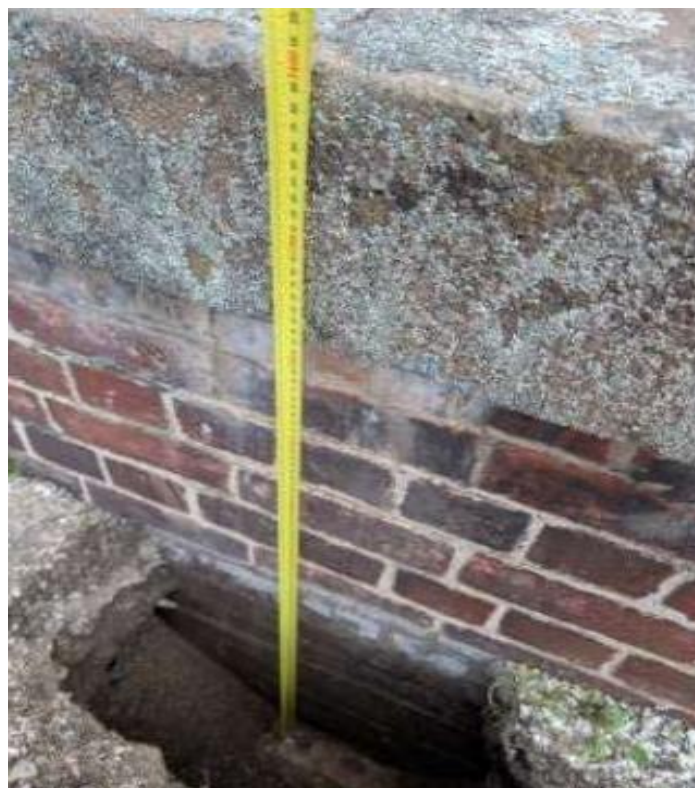
Fig.5. Rear of Platform 2 to be rebuilt.
