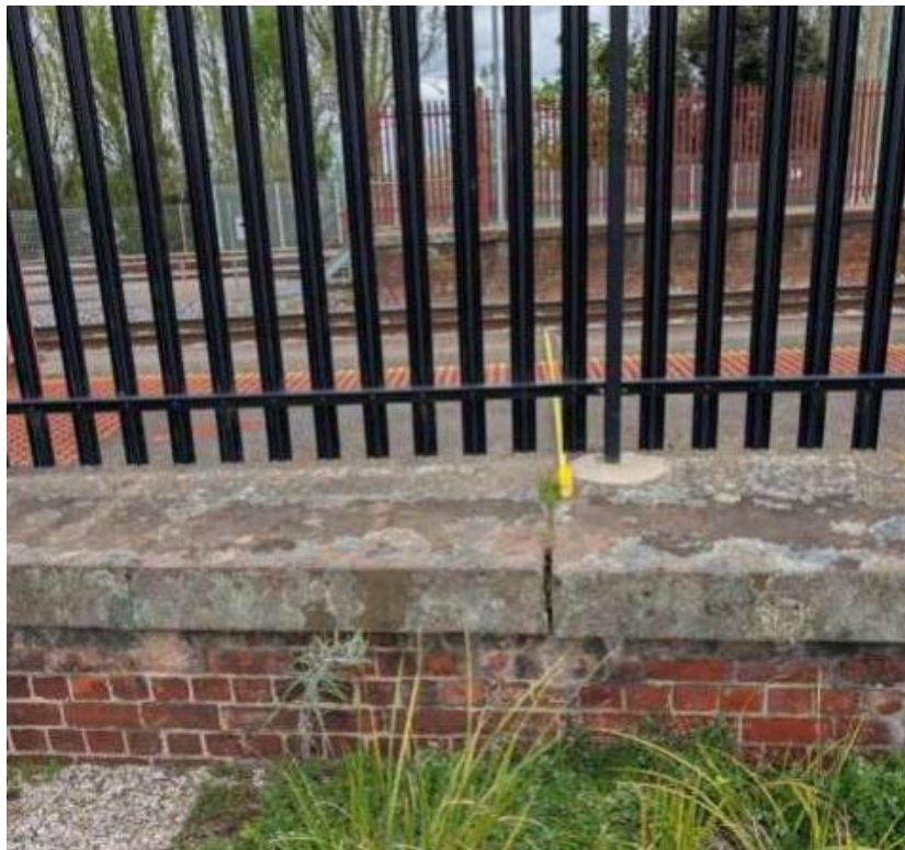
Fig.5. Rear of Platform 2 to be rebuilt.
