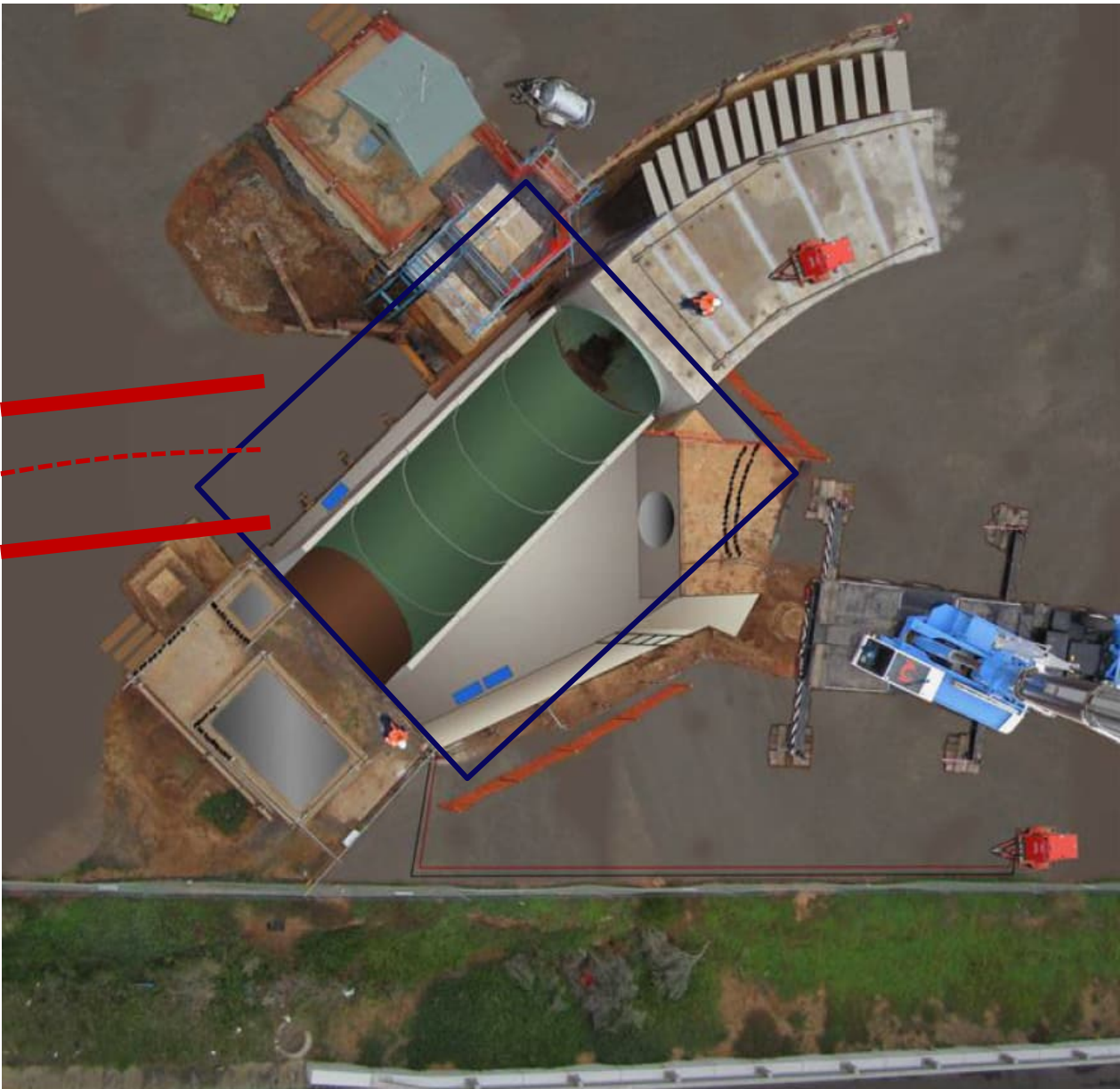
Figure 4. Image during construction of WTS, showing the proposed location of WTS006 shaft (blue square) and the approximate location of the possible remainder of the MOS (red lines) not removed during WTS construction
