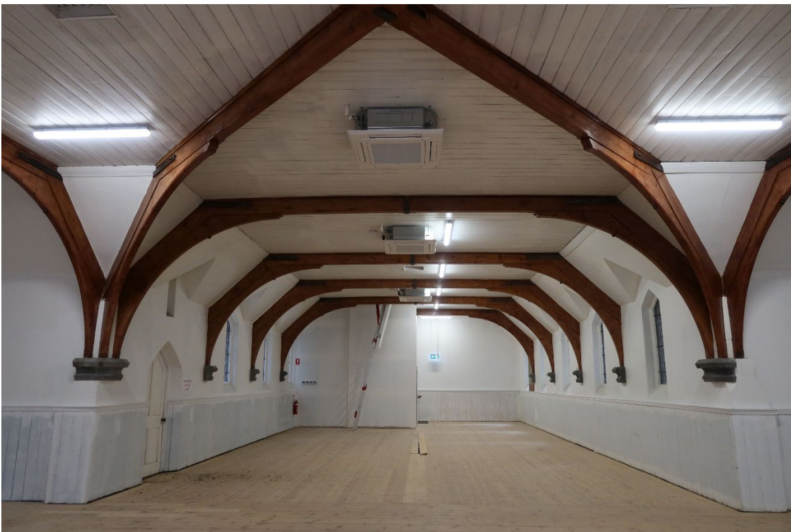
Figure 6 First floor north wing, looking north toward the lift (rear, at left); note exposed roof trusses and timber lined ceiling
