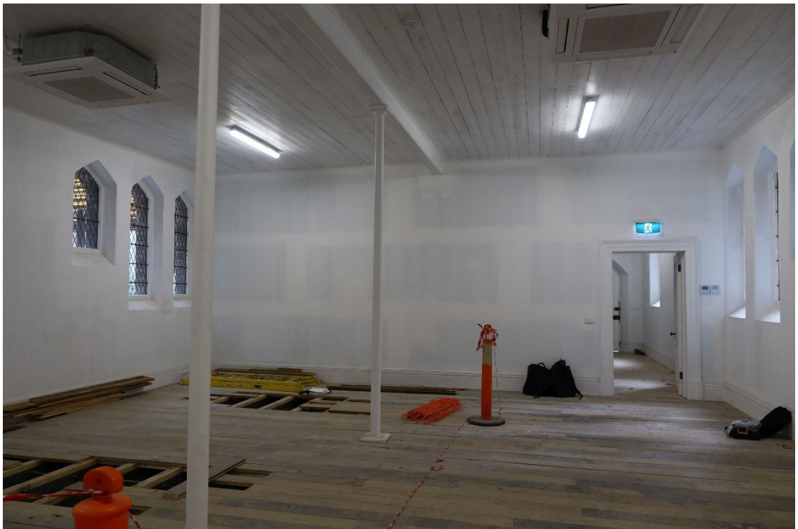
Figure 4 North wing ground floor, viewing to the north; the modern wall separates the lift/stair from this space
