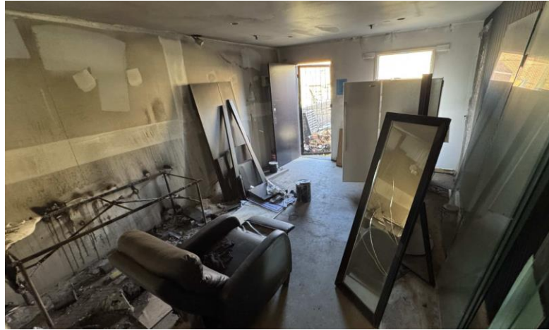
Figure 38: View of the third premise from the north, rear room that had undergone partial refurbishment. Source: Trethowan Heritage, 2026.
