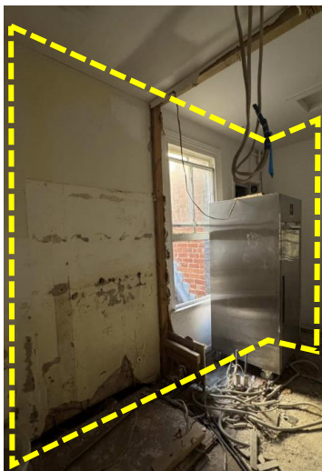
Figure 50: The walls outlined in yellow may potentially be original/early. They are on the mezzanine floor. Source: Trethowan Heritage, 2026.
