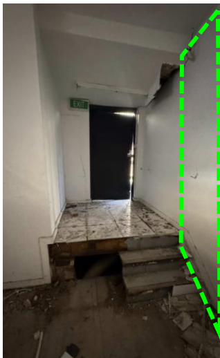
Figure 51: The wall outline in green may potentially be original/early. It is located on the mezzanine floor. Source: Trethowan Heritage, 2026.
