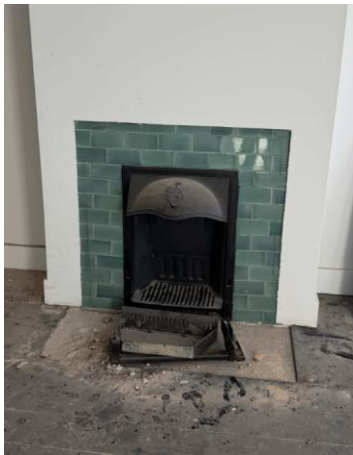
Figure 39: View of the fourth premise from the north, exposed fireplace. Source: Trethowan Heritage, 2026.
