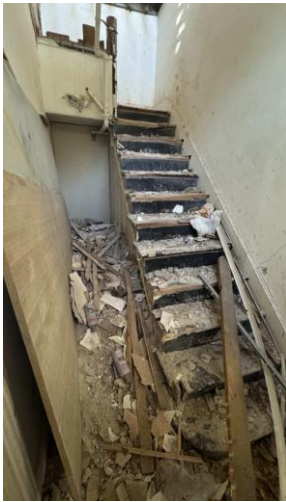
Figure 21: View of northern terrace, one of the central rooms with dilapidated timber staircase. Source: Trethowan Heritage, 2026.
