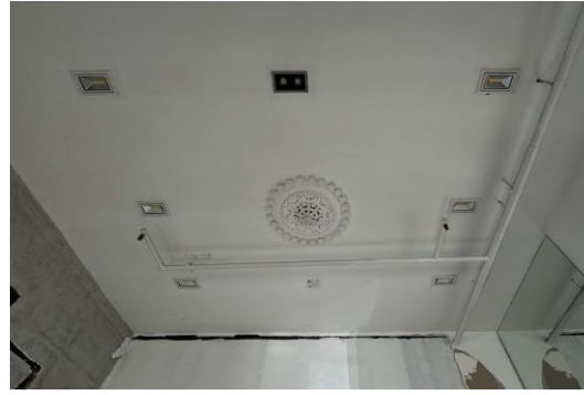
Figure 20: View of the northern terrace, easternmost (front) room ceiling. Source: Trethowan Heritage, 2026.
