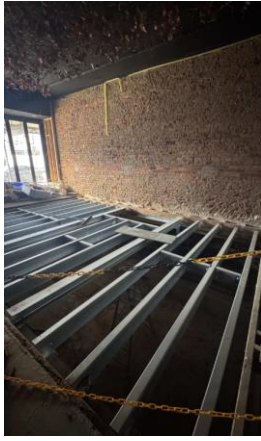
Figure 27: View of the southern terrace's south wall and floor cavity. Source: Trethowan Heritage, 2026.
