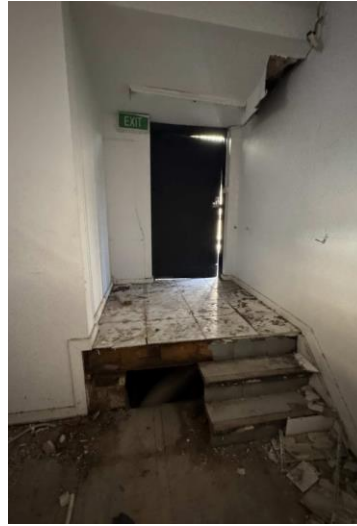
Figure 45: View of the western wall and door at the mezzanine floor. Source: Trethowan Heritage, 2026.
