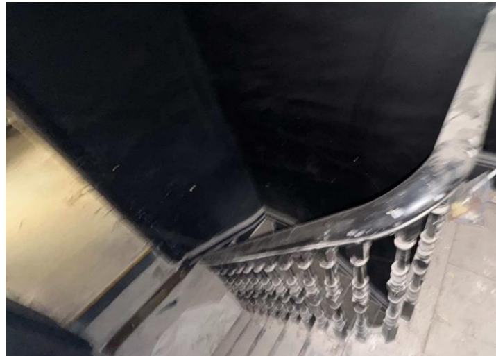
Figure 43: View of the timber staircase at the rear of the southernmost premise. Source: Trethowan Heritage, 2026.
