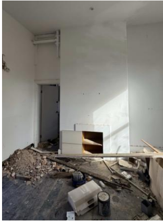
Figure 34: View of one of the northernmost premise's chimney breast and fireplace, now converted into shelves. Source: Trethowan Heritage, 2026.
