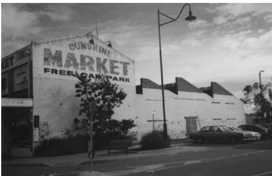
Figure 5. View of the east elevation of the Sunshine Market, c2000 (Source: Victorian Heritage Database)
