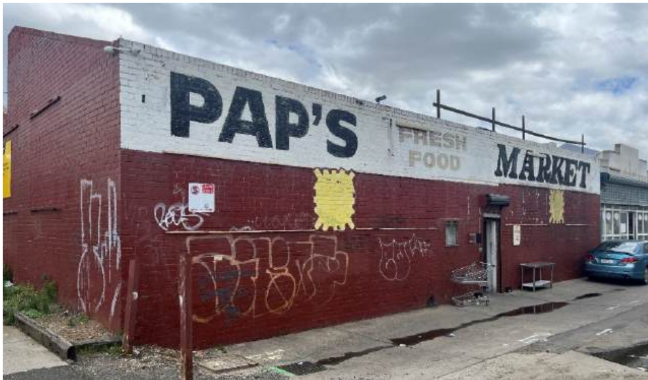
Figure 10. View of the rear (north) elevation of the Former Sunshine Market building (Source: GJM Heritage, November 2025)
