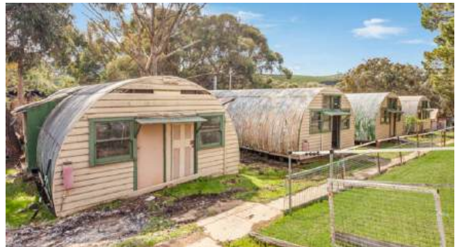
Figure 48. Nissen huts, part of the Former Our Lady of the Ark, Morningside Commune, Tyaak. (Source: realestate.com.au)
