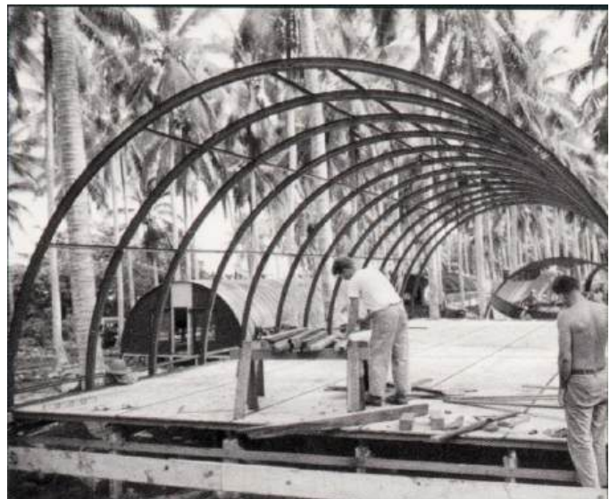
Figure 7. (above) Constructing officers' quarters, Russell Island, South Pacific, 10 November 1943. (Source: Quonset Hut – Metal Living for a Modern Age, p 65)
