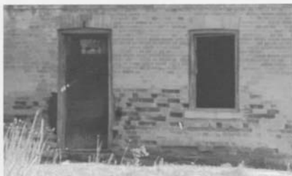
Poor maintenance has resulted in damage and deterioration to this building.
