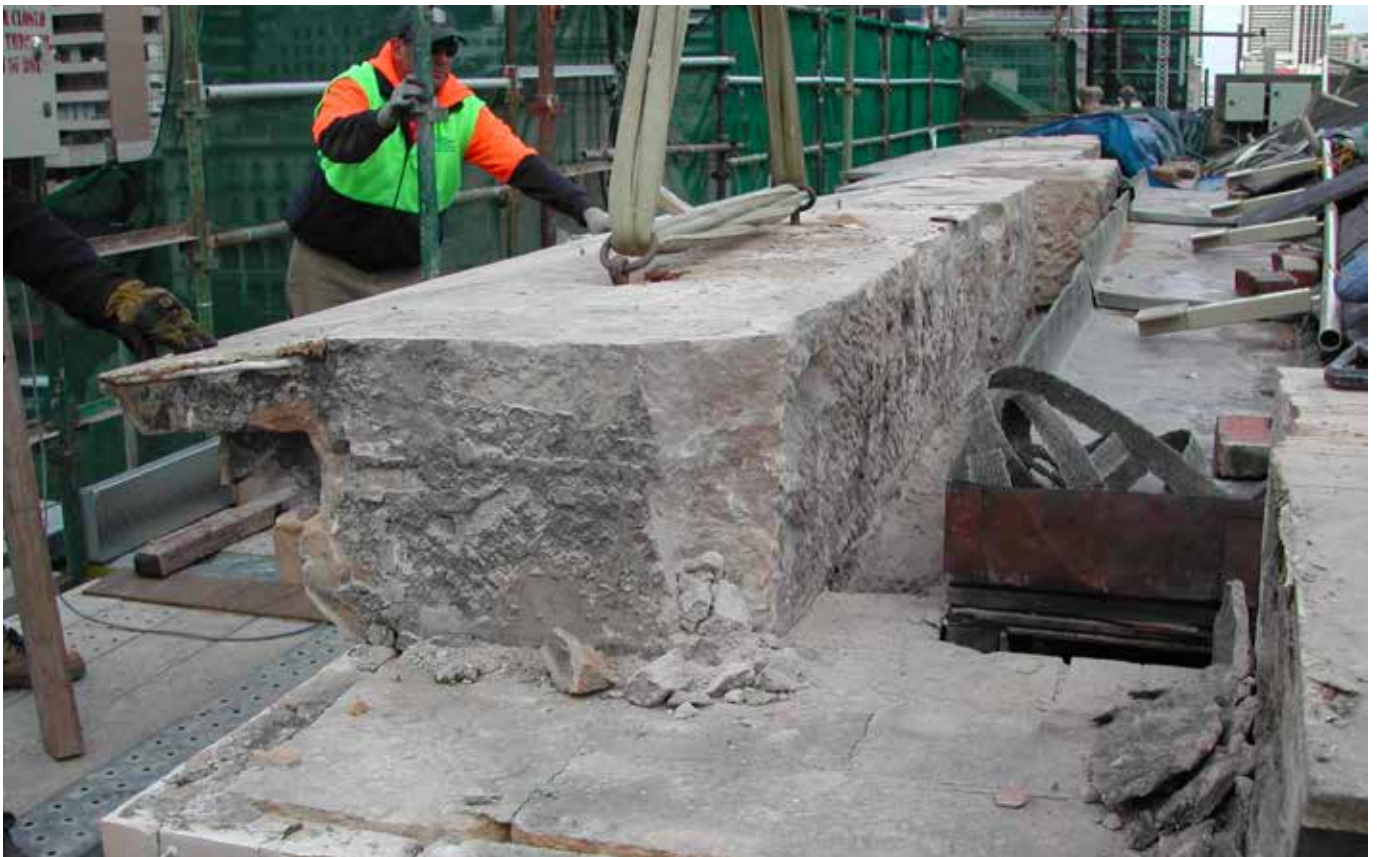
Parliament House, Melbourne Conservation works to Parliament House including extensive parapet reset works completed along the south and east facade. The removal of the cornice course exposed the thin veneer of previously completed repairs that, in most cases, exceeded their life expectancy requiring remediation works. The deterioration of the previous veneer repairs was amplified by the ingress of water through the cornice joints causing the fixings to rust and the stone to decay internally, which resulted in the repairs becoming unsound.
