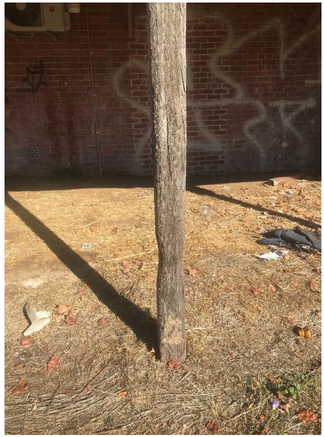
Figure 24 – Weathered timber post.
