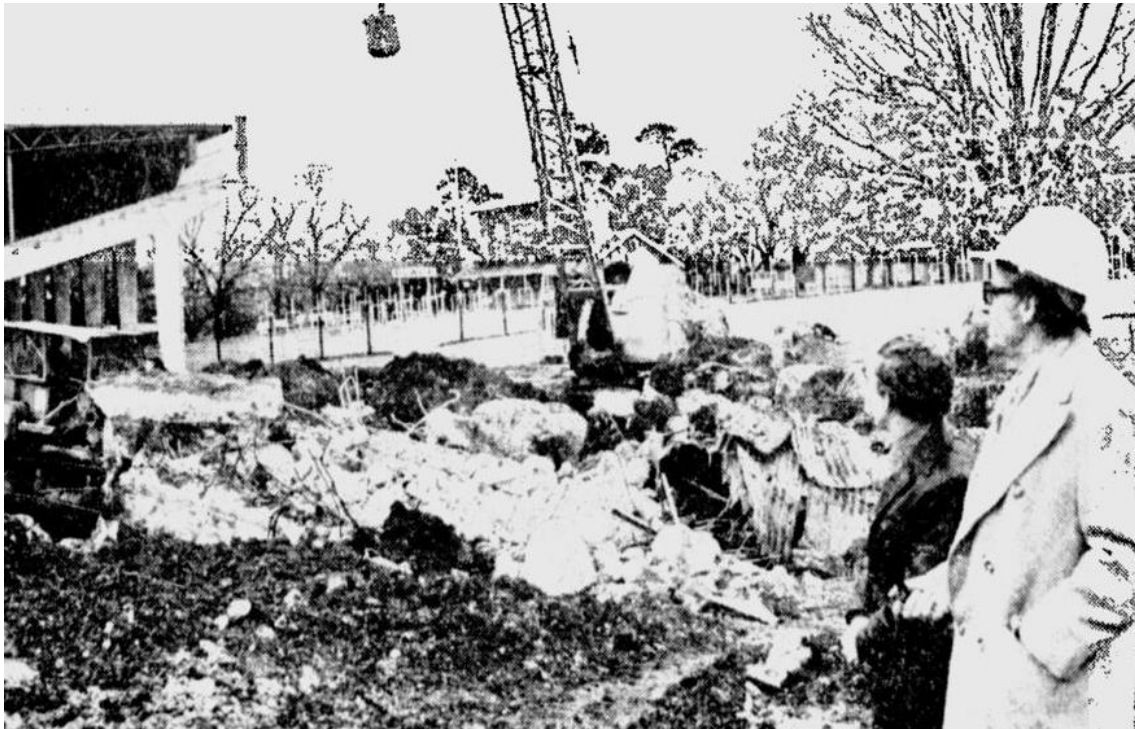
Figure 28 Demolition of the old Hill Stand to make way for the new five storey grandstand. Source: The Age , 15 June 1977, p. 12.
