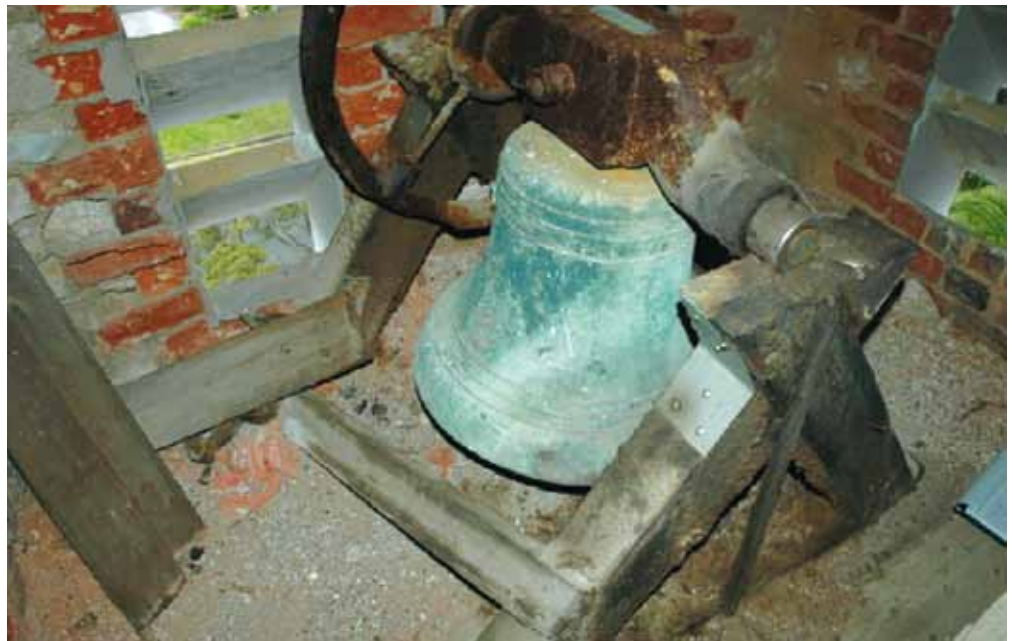
Figure 26: Bell and associated system in the tower of St. George the Martyr Anglican Church, Queenscliff, 2005. Source: Wendy Jacobs and David Rowe.
