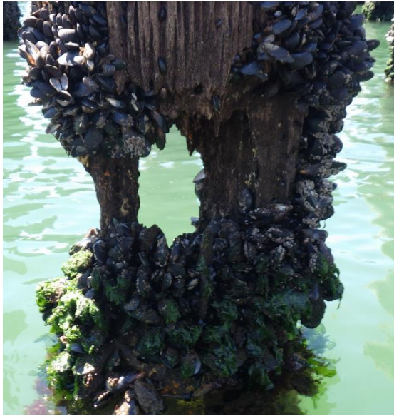
Figure 4. Failing pile – hollowing (104-E)
