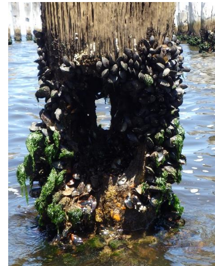
Figure 7. Failing pile – hollowing (168-W)
