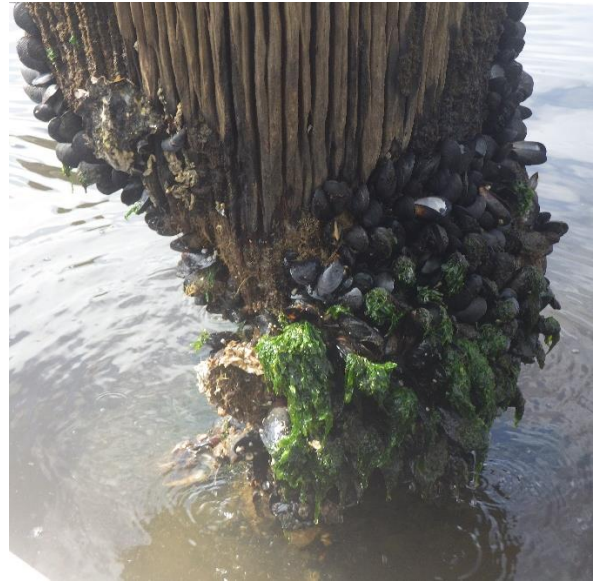
Figure 5. Failing pile – necking (148-L)
