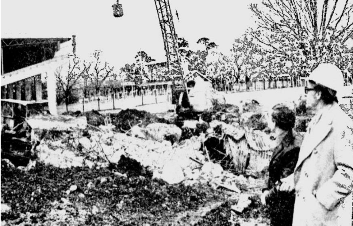
Figure 28 Demolition of a portion of the 1957 Hill Reserve Stand to make way for the new five storey grandstand Source: The Age , 15 June 1977, p. 12
