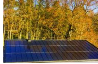
RF01 SOLAR PANEL ROOF
