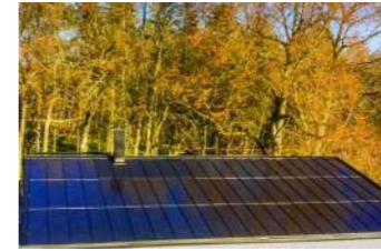
RF01 SOLAR PANEL ROOF
