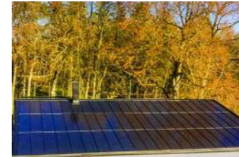
RF01 SOLAR PANEL ROOF
