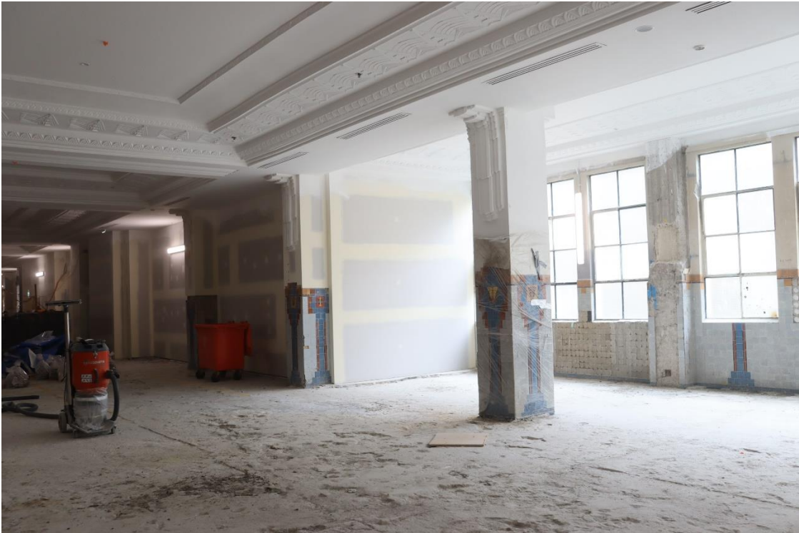
East wall alcove - wall tiles and plaster capitals to be reinstated/fabricated
