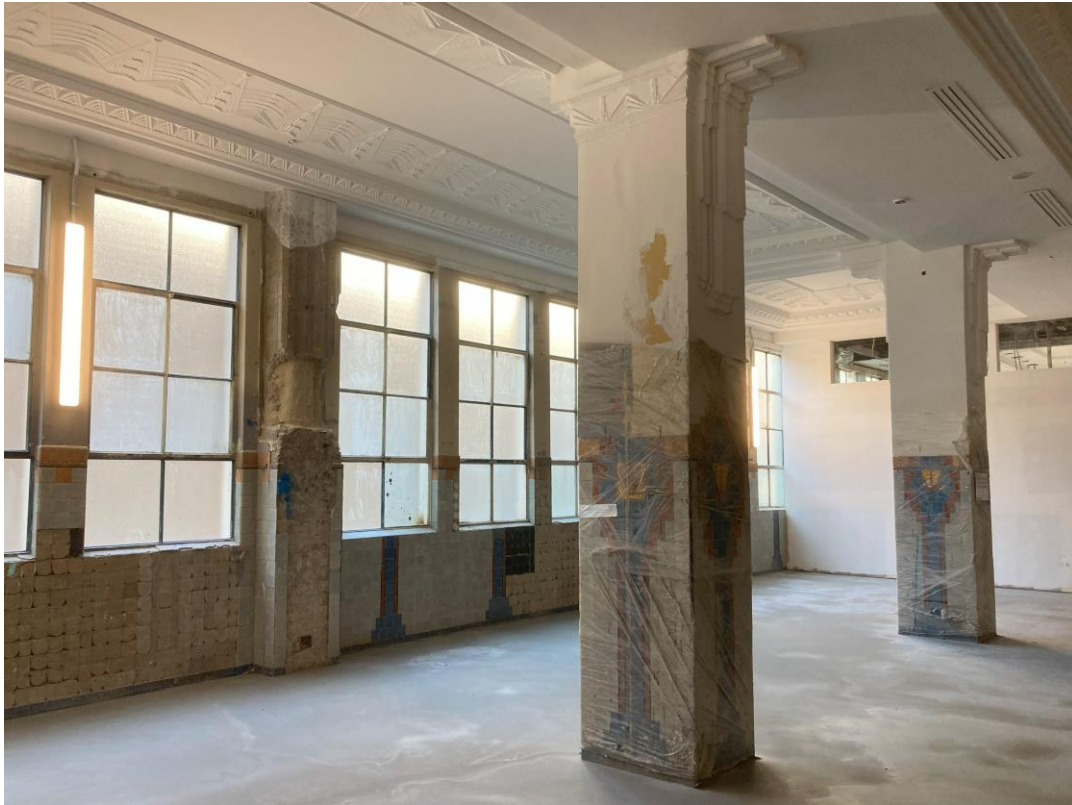
East wall alcove – wall tiles and plaster capitals to be reinstated/fabricated
