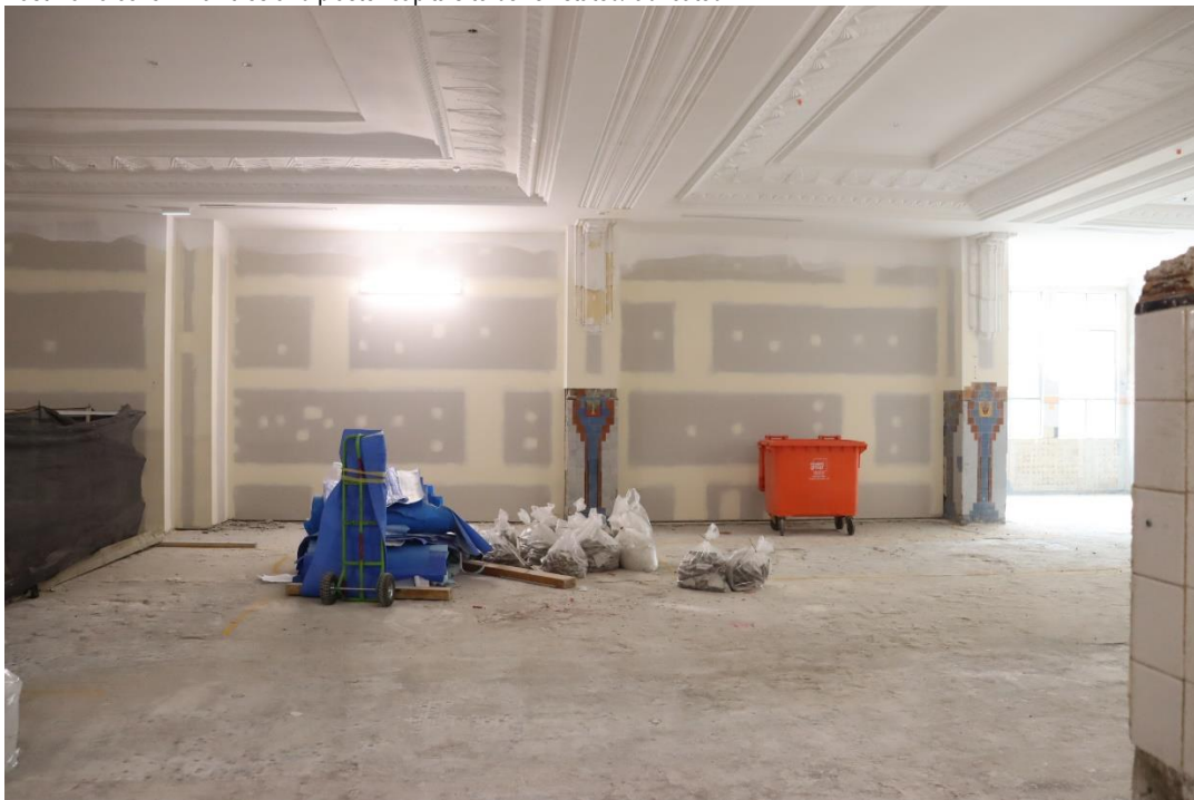
East wall between grid lines 7 and 9 – tiles to be reinstated/fabricated
