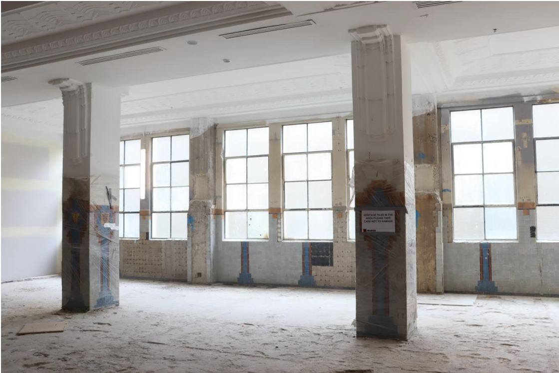
East wall – tiles to be reinstated/fabricated
